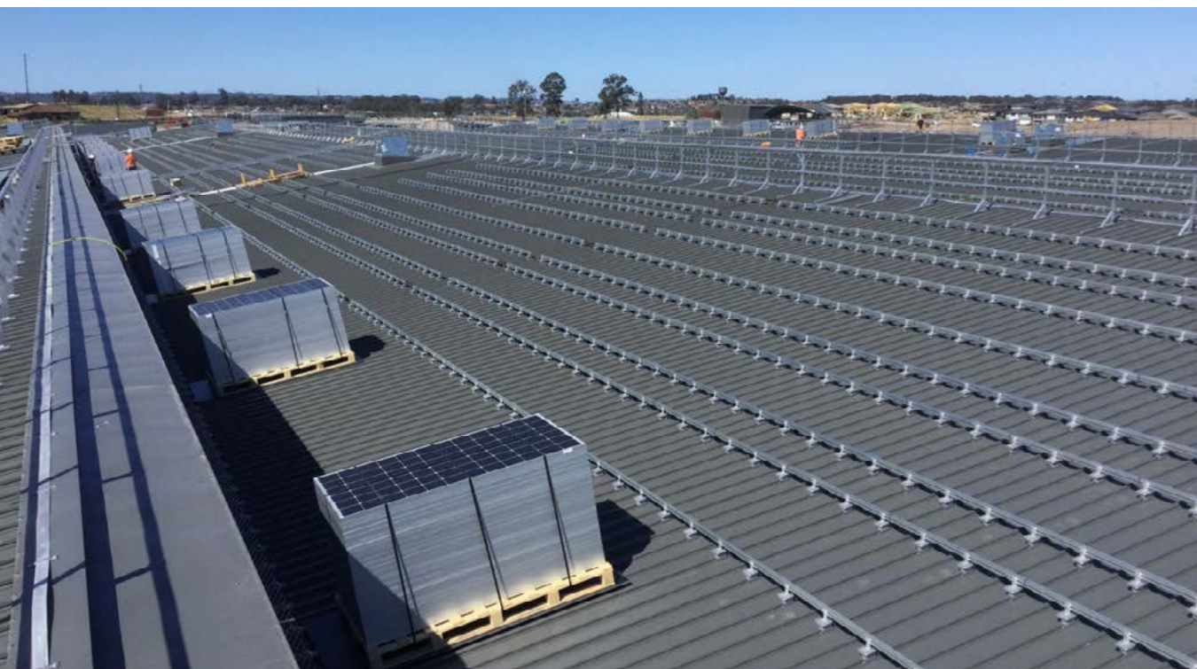
Preparing the roof of the Sydney Metro Trains Facility to install the 1.1 megawatt (MW) solar array
