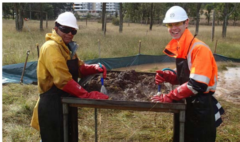
Sieving excavated material for Aboriginal artefacts as part of the Sydney Metro Northwest program
