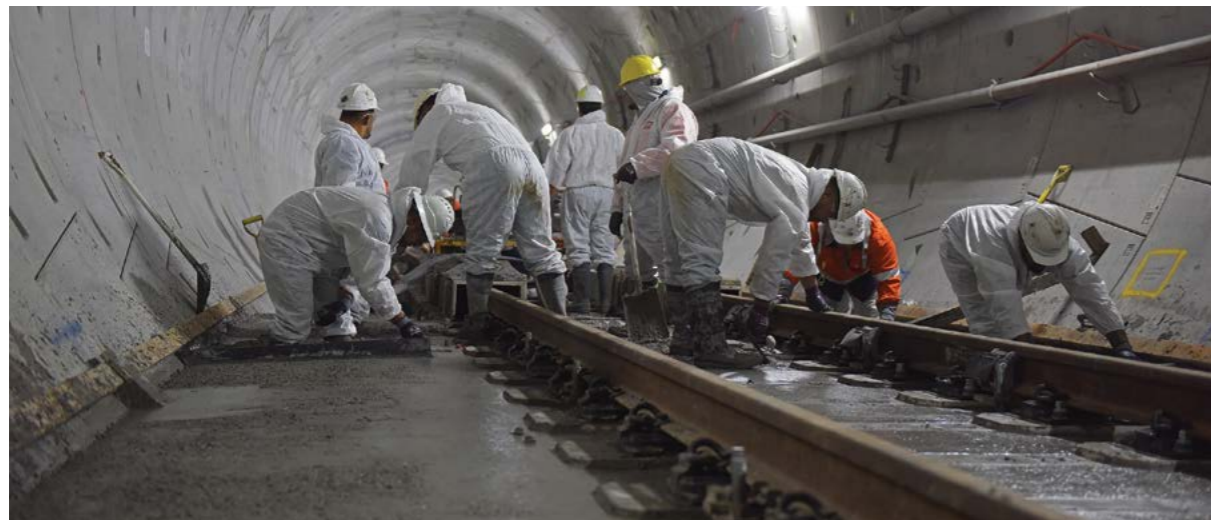
Workers 21 metres under Norwest Boulevard at Bella Vista; concreting metro railway tracks in the city-bound tunnel
