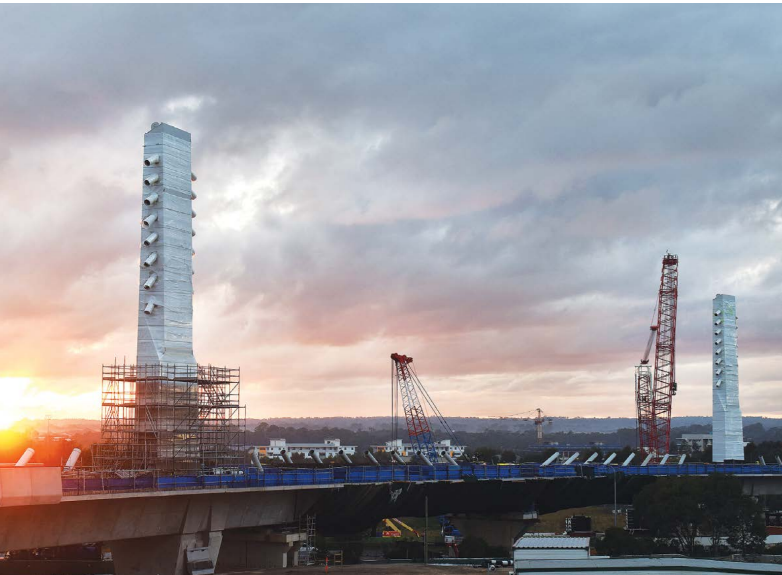
Dawn on 28 May 2017 - the first morning where both bridge towers over Windsor Road were in place. The bridge is constructed to with stand identified climate risk.
