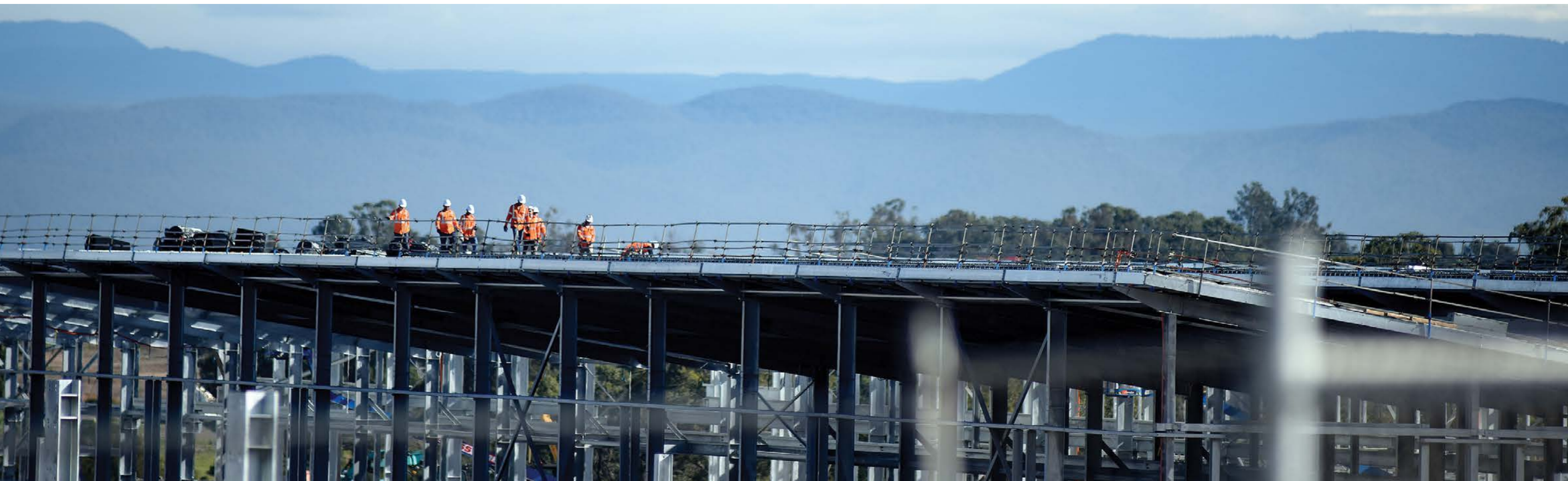
Workers on site at the Sydney Metro Train Facility under construction at Cudgegong Road.
