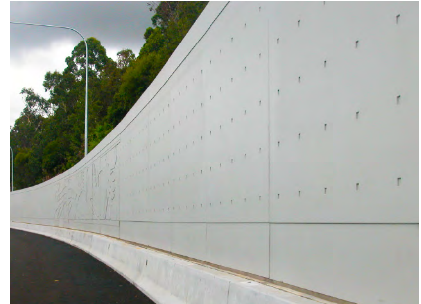
Gore Hill Freeway, Sydney. Provide retaining walls that are topped out by a consistent concrete capping beam. Source: AECOM.
