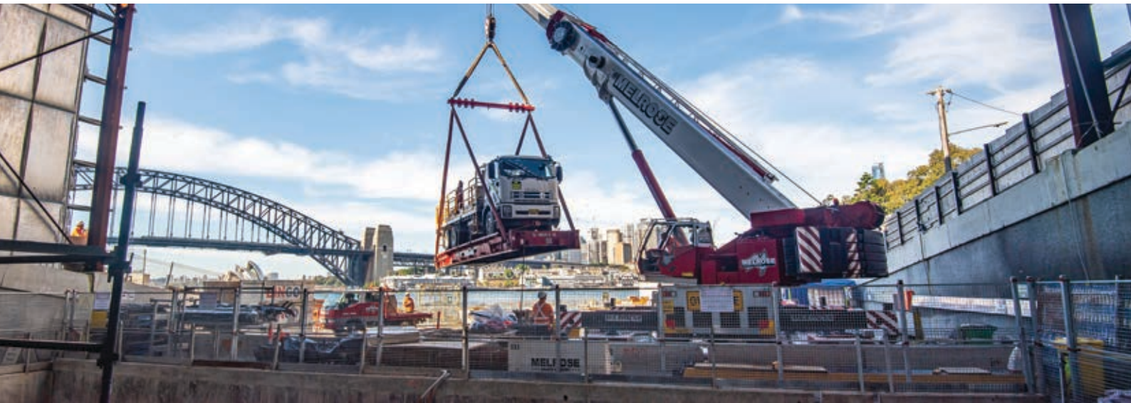
Hi-rail truck being delivered into the tunnel to continue fit out work.
