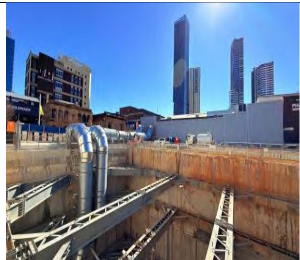
Figure 2.4: Vent fans installed, adjacent to Western end of Station Box.
