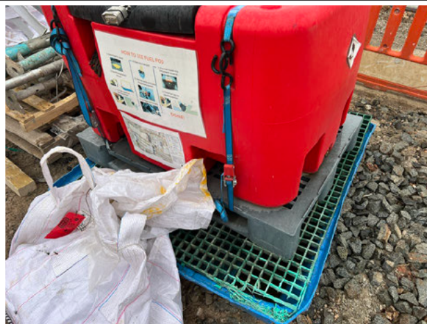
Compound: There was liquid in the fuel pod bund.
