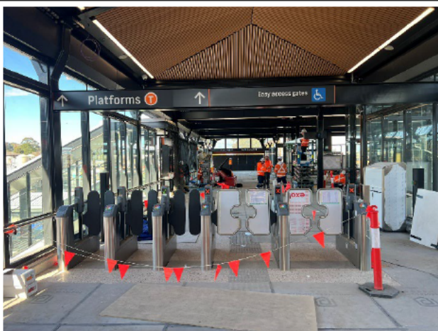
Overpass: The ticket gates have been installed successfully.
