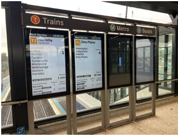
Overpass: Electronic sign boards have been installed and are synced with the ones on the platform.
