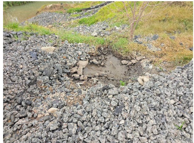
ORHN - Basin rock check required maintenance following street-sweeper washout.
