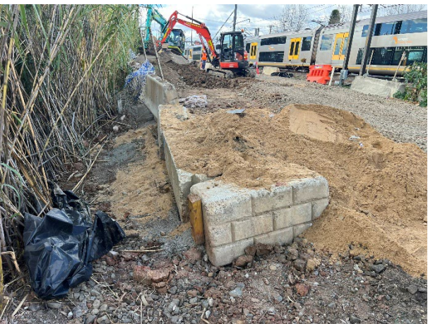
Laydown area 1: Minor amounts of sand have spilt over the jersey barriers, however remained within the site boundary.
