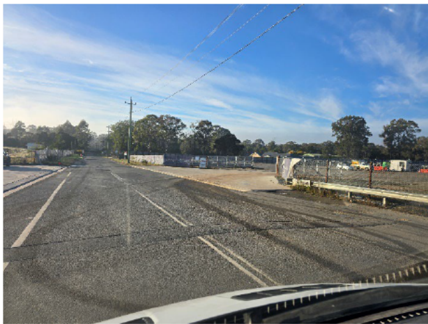
Lansdowne Rd to Patons Lane – Minor tracking onto Lansdowne Rd.
