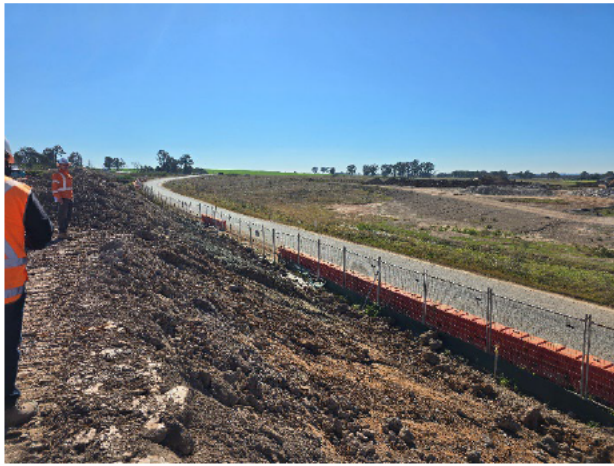
BRD – Batter ESC was required at Innovation East.
