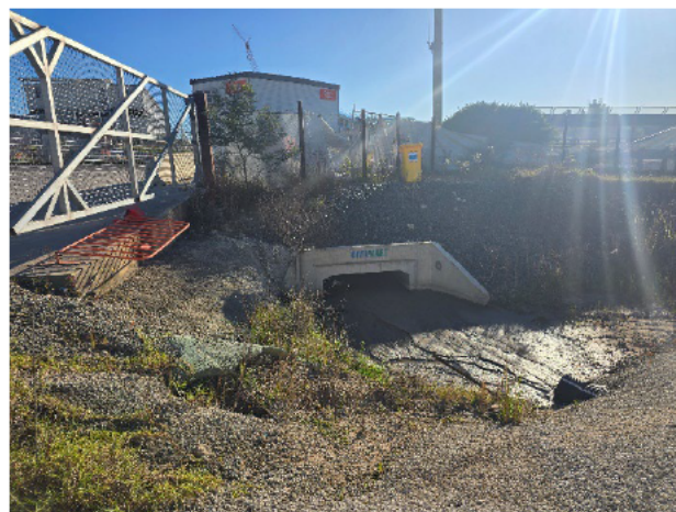
ORH – sediment buildup in culvert sump.
