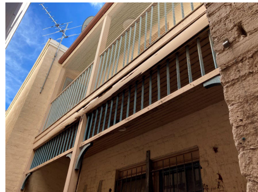
Figure 2.31: Detail view of rear balcony prior to demolition. Note non-traditional details and extensive termite damage. The two-storey toilet block addition is partly visible to the left of the image. Source: OCP Architects, 21 April 2022.
