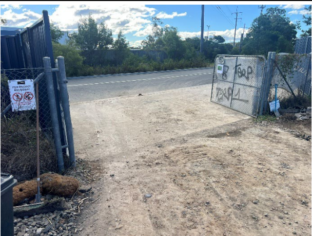
Laydown area 1: Mud tracking was observed at laydown area 1.
