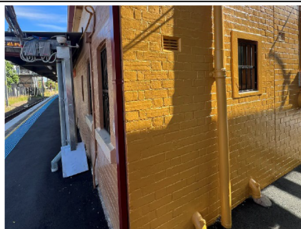
Platform 3/4: The paint on the platform building is not a match to the existing, and the project is working with heritage specialists to identify an acceptable colour.
