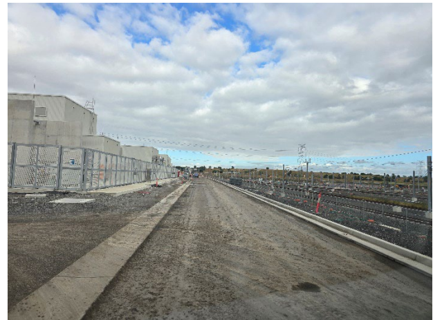
SMF – Transformers and rail lines.
