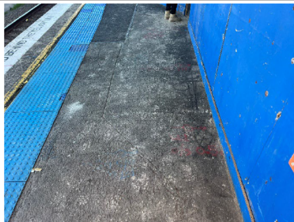
Platform 3/4: Mud was tracked from within the hoarding to the platform.
