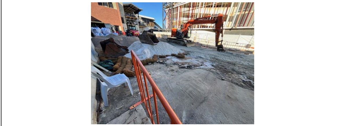
Photos 6-8: Northern plaza – CSR installation.
