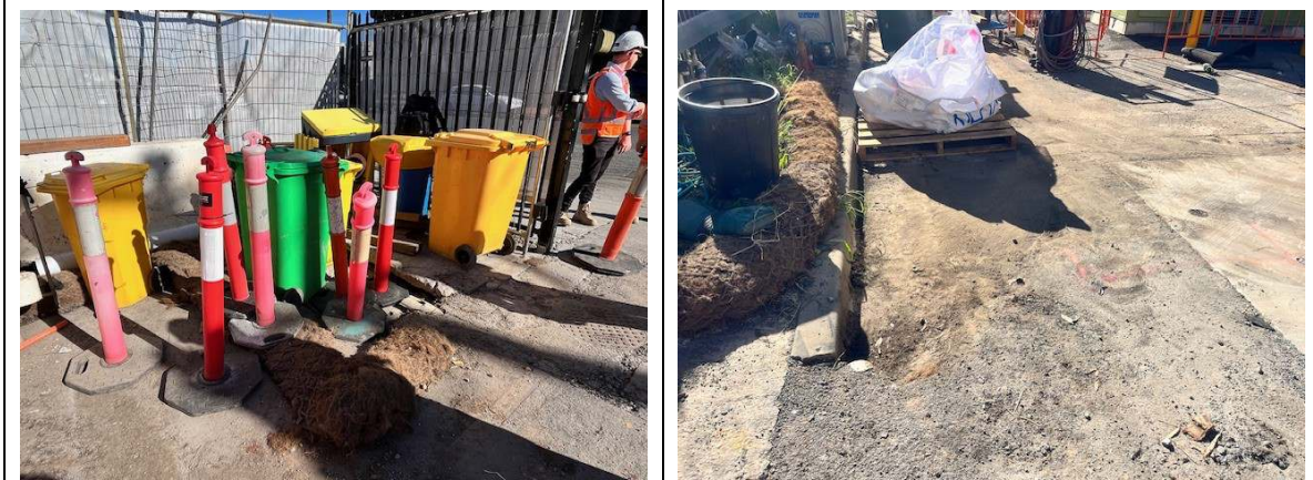
Photos 9 & 10: Missing and deteriorated ERSED controls around the stormwater drain adjacent to the Northern Plaza CSR works.
