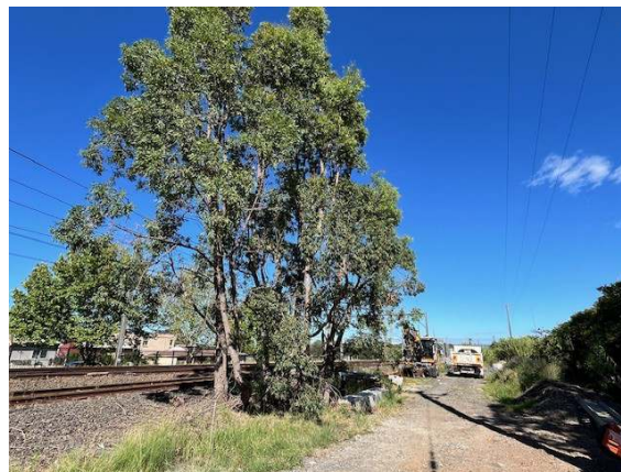
Photo 21: No tree protection established around the tree in Laydown 1.
