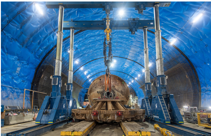
An underground gantry crane and self-propelled modular transporter (SPMT) is used to transport pieces of the TBM through the station cavern to the Hunter Street East shaft.
