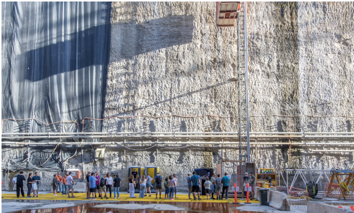
Community members accessed the tunnel via an Alimak (construction elevator), entering and exiting through The Bays station box.
