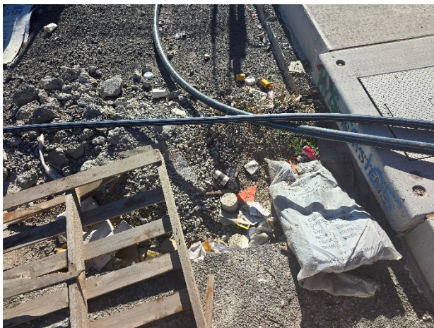
SMF – Litter and waste removal was required.
