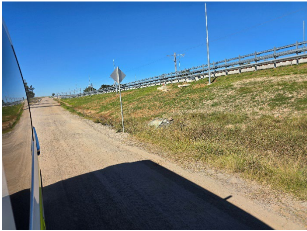
Luddenham to M12 – Coir log maintenance in drainage swales was required.
