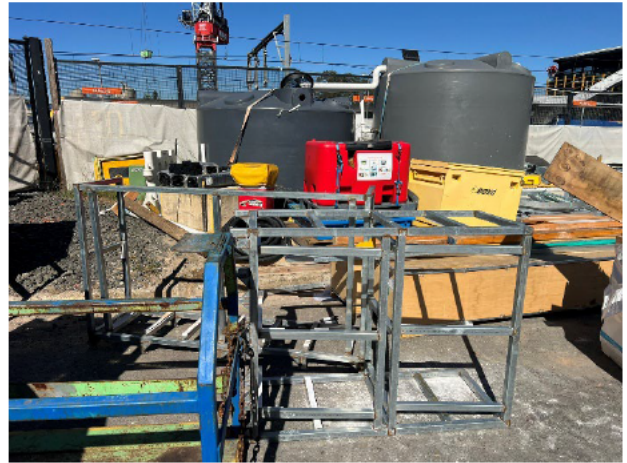
Compound: The spill kit at the refuelling area was obscured by construction material.
