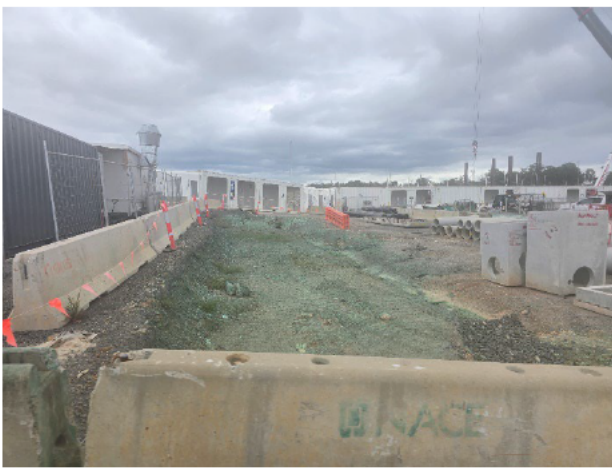
BRD – Sediment accumulation around swale sandbags.
