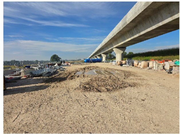
LUD – Haul Road required maintenance in several areas.
