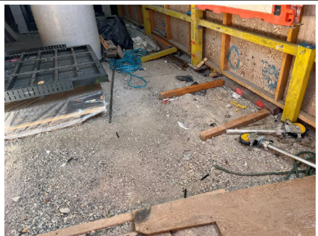
Platform 3/4: Litter was observed in the area enclosed by hoarding.
