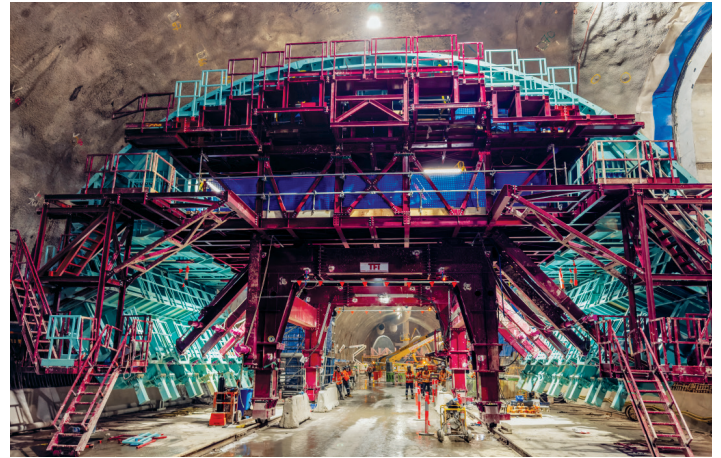
About 24,000m 2 of waterproofing membrane was used to complete the roof of the cavern.
