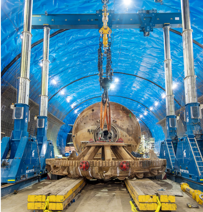
An underground gantry crane and multi-service vehicle is used to transport pieces of the TBM through the station cavern to the Hunter Street East shaft.
