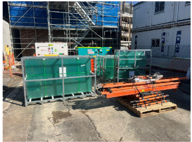
Compound: Glass panels to be installed in the overpass are stored adjacent to the Sydney trains building.
