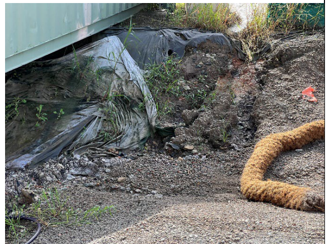
LUD – ESC required maintenance post storm event.
