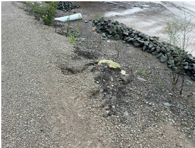
OHE – Erosion of the Kent Road batter post storm required repair and cleanup of haul road.
