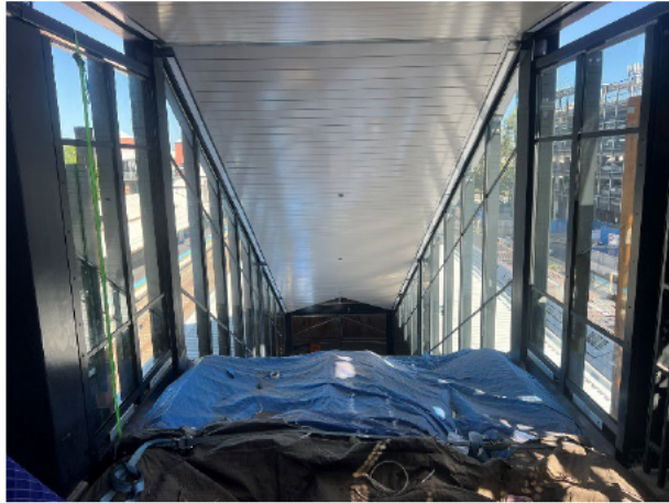
Overpass: Escalator works are due to commence as the glazing is complete in the void.
