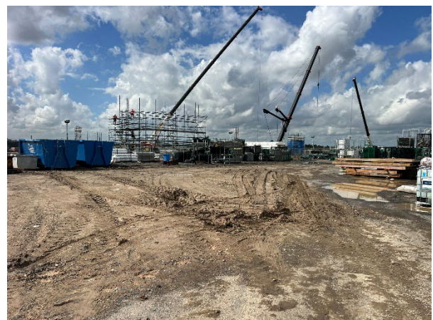
BRD – Haul road required reinstating.
