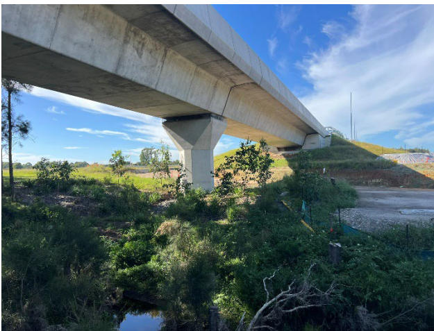
Luddenham to M12 – Cosgroves Creek pads remained intact, with no impacts observed following the rain events.
