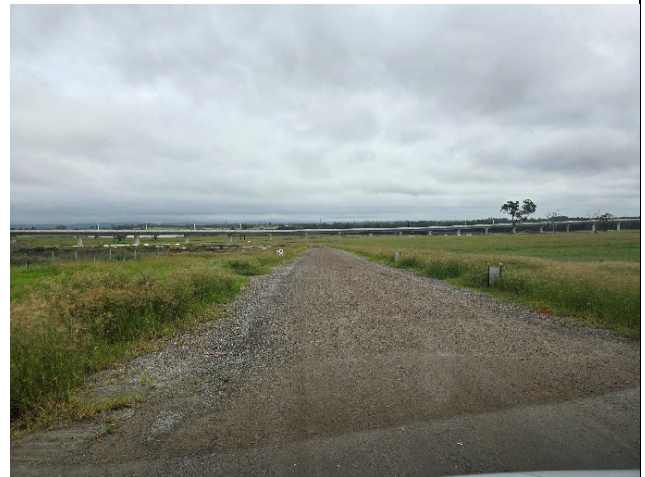
Water Pipeline to Luddenham Station – Internal haul road and stockpile area was maintained.
