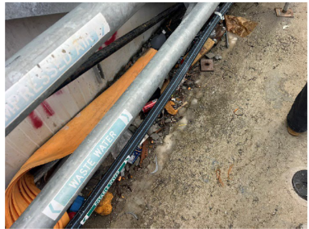
STM – litter accumulated along walkways.
