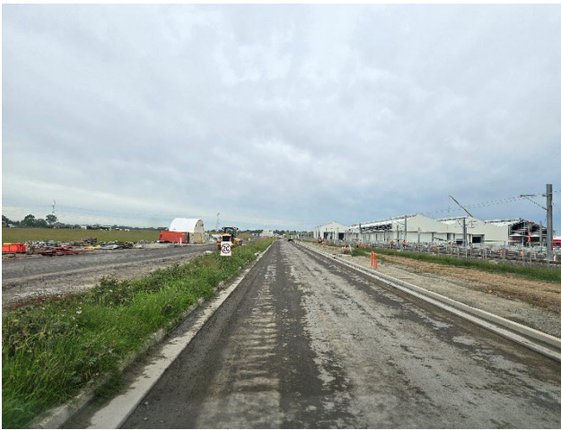
SMF – Dust suppression on haul road was observed. Track and OCS installation to the right.
