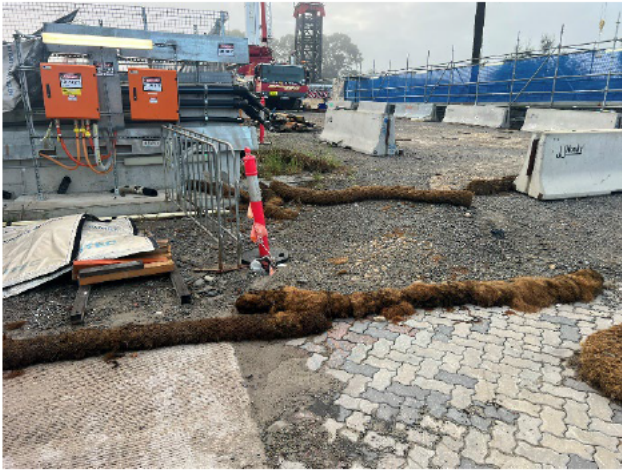
STM – Maintenance of ESC was required.
