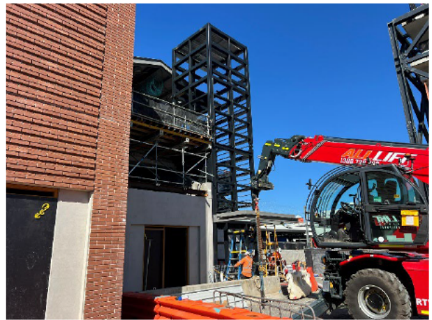
Compound: The lifting operation from the compound to the overpass continues to be effective.
