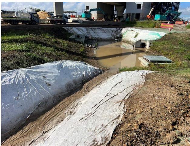
LUD – Geofabric installed after controls noted not to be installed, additional controls recommended by the ER.
