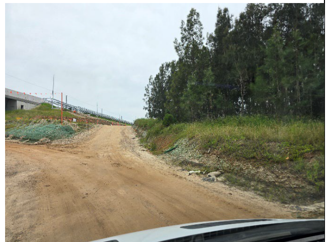
Luddenham to M12 – Reinstatement of ESC required and completed prior to the rain event.
