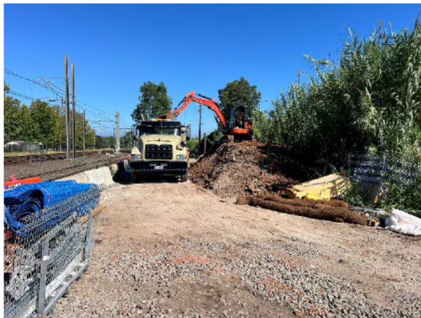
Laydown area 1: Spoil load out was occurring with the required controls in place.
