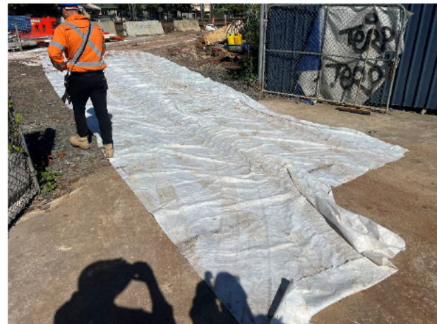
Laydown area 1: Geofabric has been placed on the haul route to minimise mud tracking on public roads.
