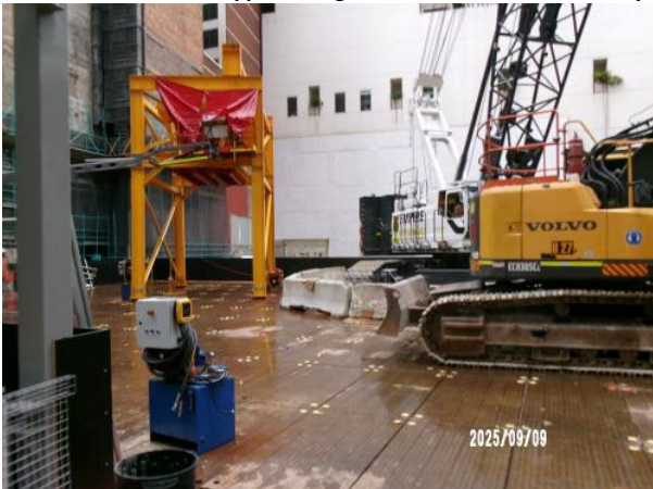
Figure 3.3 Hunter St West: Steel deck construction complete. Crane established on steel deck and in use. Kibble loading frame installed.
