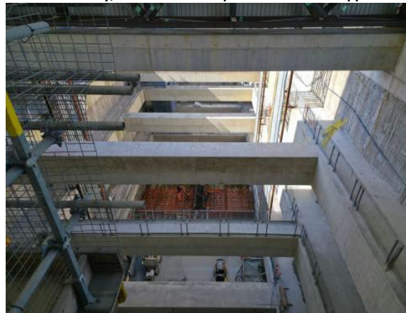
Figure 2.6 – Rosehill Site: Base slab FRP works in progress at the time of inspection.
