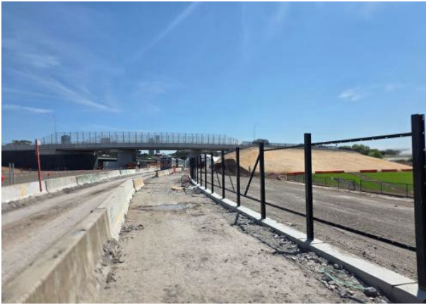
Figure 2.7 – Clyde MSF: Security fence installation and landscaping works continuing around flood basin.
