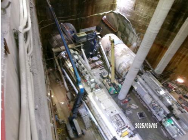
Figure 3.5 Pyrmont East: TBM Ruby had started tunnelling in the previous week and was 3 rings into rock. TBM Jessie was in place in the Nozzle having completed the traverse through the shaft. The profiler was operating in the caverns with spoil being removed to the Bays.
