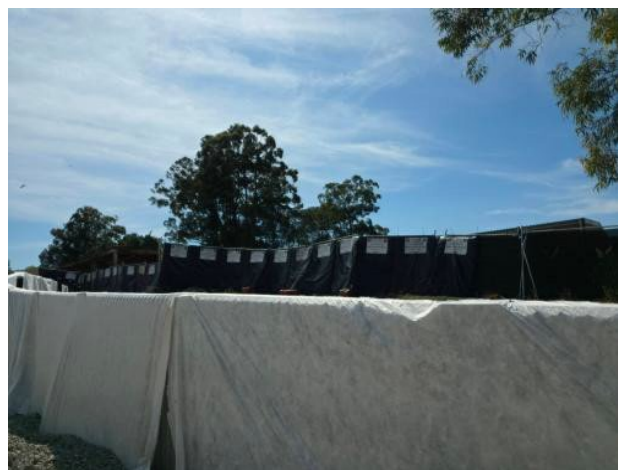
Figure 2.12 – Clyde Dive: Retaining wall with pre-cast panels installed along section of ATC boundary.
