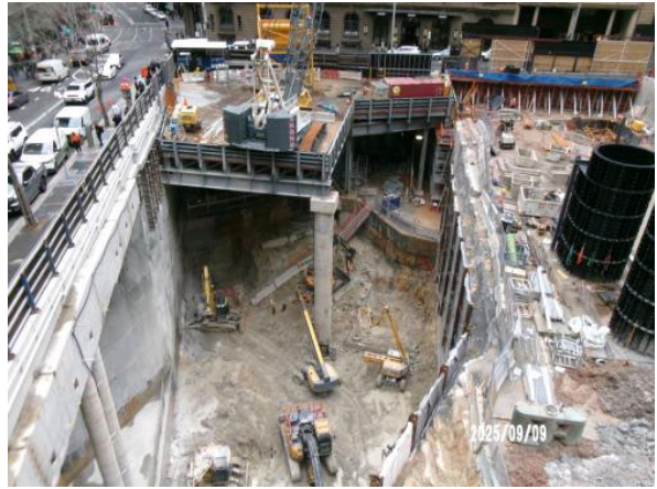
Figure 3.2 Hunter Street East: Excavation adjacent Hunter Street and load out of spoil from the steel deck.
