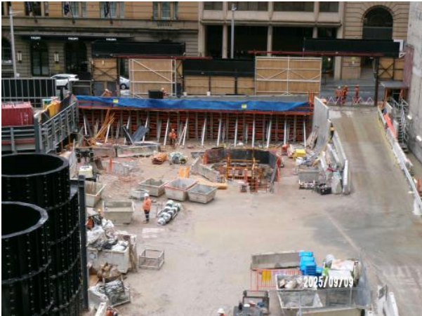
Figure 3.1 Hunter Street East: Former Acoustic Shed area. Ongoing works related to wall support along the O'Connell Street boundary.
