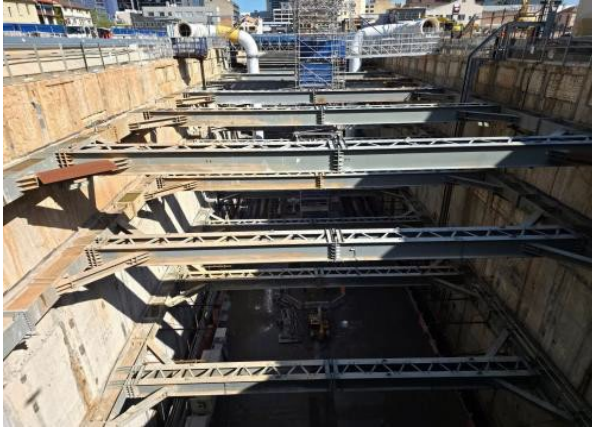
Figure 2.1- Parramatta Site: Vent fans installed in operation.
