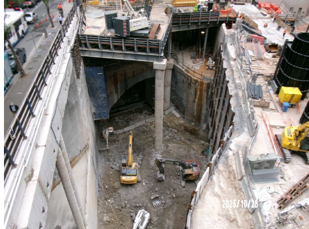
Figure 3.2 Hunter Street East: Ongoing excavation adjacent Hunter Street and load out of spoil from the steel deck.
