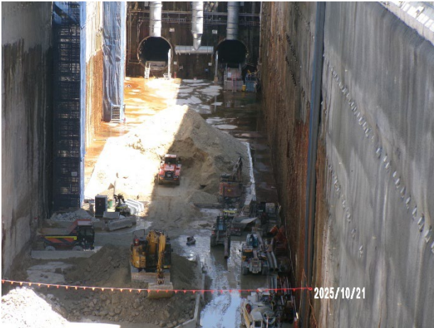
Figure 3.9 The Bays: A spoil stockpile area has been set up in the CTP side of the station box to manage spoil from the Pyrmont site.
