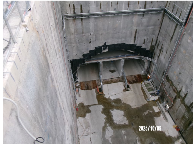
Figure 1.6 Automatic pumping systems were observed to be working (Burwood North).
