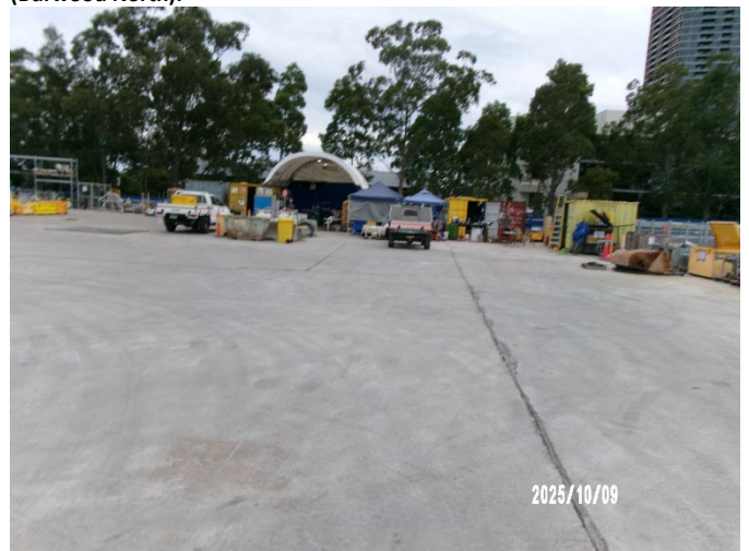
Figure 1.8 Ongoing consolidation and removal of plant, equipment and materials at the surface (SOP).
