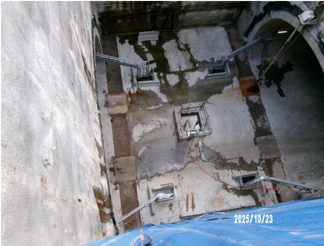
Figure 1.3 Eastern Shaft – Base of the eastern shaft. Automatic water management system operating (Five Dock).
