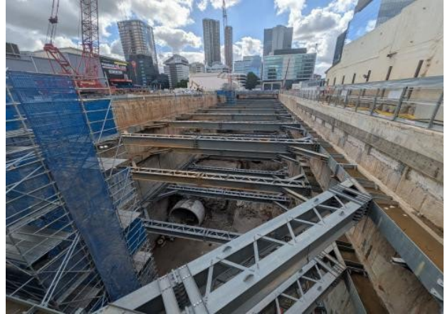
Figure 2.2 – Parramatta: Western Station Box - no hammering works at the time of the ER Inspection; material load out observed.
