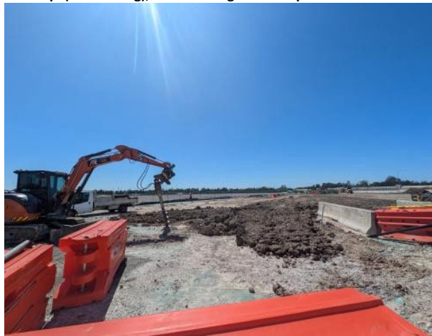
Figure 2.9 – Clyde MSF (West): Portion 12B backfilling of previous crib and site office area complete – treated PASS placement ongoing.
