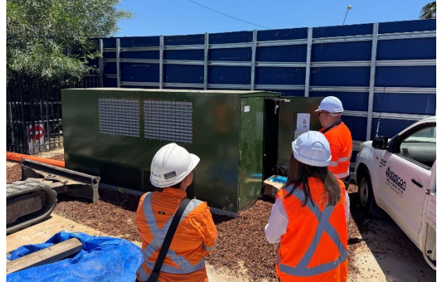
Figure 5.2 ER Inspection / DPHI Site Visit. Cable terminations being undertaken within Kiosk. Discussed alterations to site hoarding at the Kiosk location, effectively implementing a noise barrier for all works on the site. Noise blankets have also been installed on the site gate.
