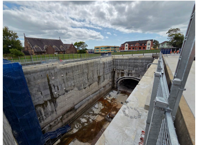
Figure 1.4 Western Shaft – no apparent works at the surface or Station Box (Five Dock).
