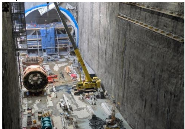
Figure 2.6 – Westmead: TBM demobilisation, formwork dismantling, cavern lining and other FRP works ongoing.
