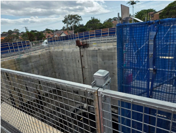
Figure 1.3 Eastern Shaft – Automatic water management system operating at the base of the East Shaft (Five Dock).
