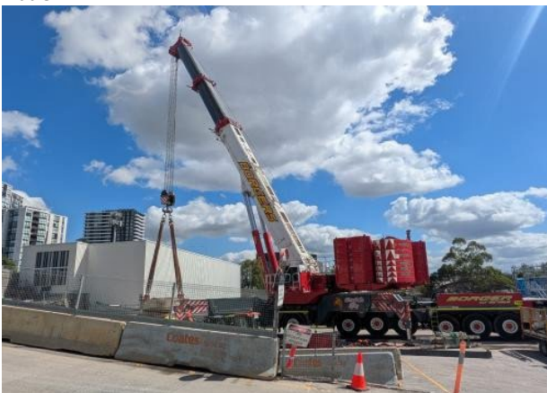
Figure 2.5 – Westmead: Surface level – Cranage underway with 750T lifting Main Drive of TBM.
