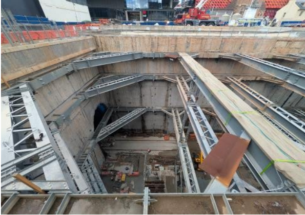
Figure 2.1- Parramatta: Eastern Station Box - GLC reports Tunnel Nozzles secondary lining and FRP works.
