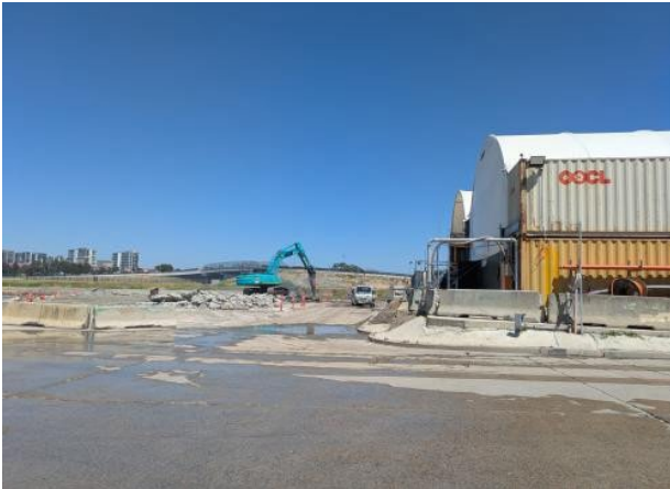
Figure 2.7 – View from Rosehill: Flood Basin Stage 2 works - concrete break up (hammering), with misting cannon operational.
