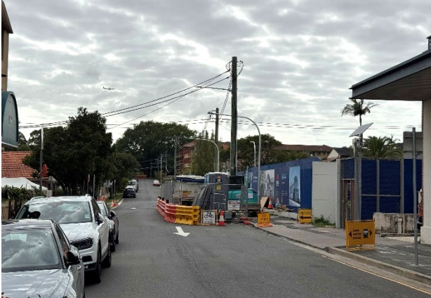
Figure 4.1 Pedestrian diversion around active work areas. Signage in place as per TGS.
