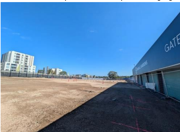
Figure 2.11 – Clyde Dive: Section of northern area, with finished levels, scheduled to be chipsealed late January 2026.
