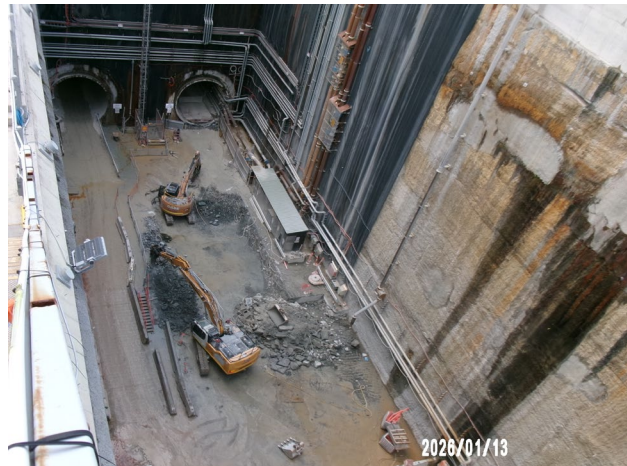
Figure 3.8 The Bays: Installation of temporary services in trenches in the Station Box.
