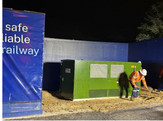
Figure 5.2 Hoarding re-configured around the Kiosk, re-instating access to public verge as required by Ausgrid standards. Ground being prepared ahead of mulch placement around Kiosk.
