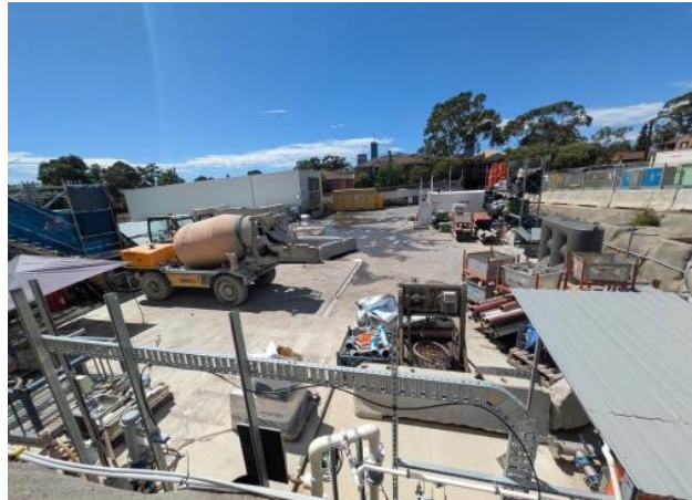
Figure 2.6 – Westmead (Surface level – Pad 3): Demobilisation / housekeeping commenced in preparation for shed demobilisation.
