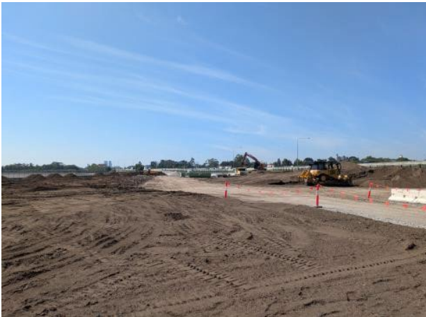
Figure 2.13– Clyde MSF: Treated PASS stockpiled material push-out and placement ongoing including commencement of topsoil placement, in preparation for landscaping.
