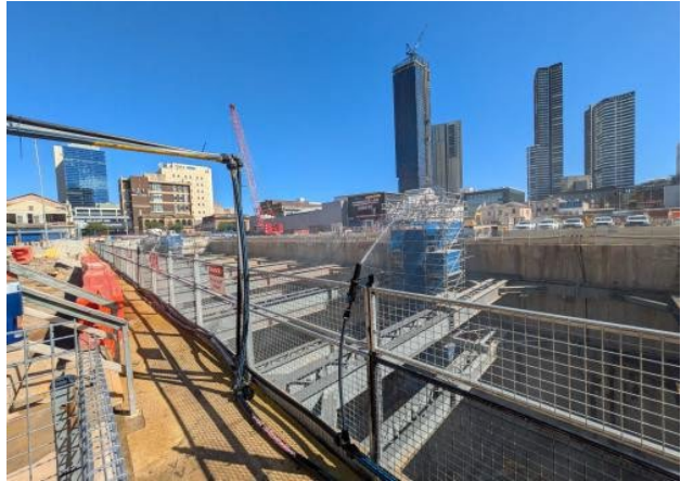
Figure 2.2 – Parramatta: Western Station Box - hammering works underway; with water misting system observed at surface level.
