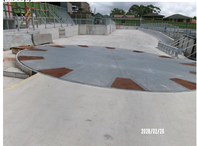
Figure 1.4 Western Shaft – no work was being undertaken at the surface or Station Box (Five Dock) during inspection.
