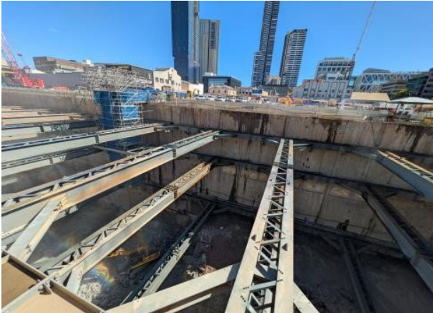
Figure 2.1- Parramatta: Western Station Box - hammering works underway within box, with water misting system observed.
