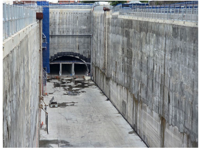
Figure 1.6 No visible activities occurring in the station box during site inspection (Burwood North).
