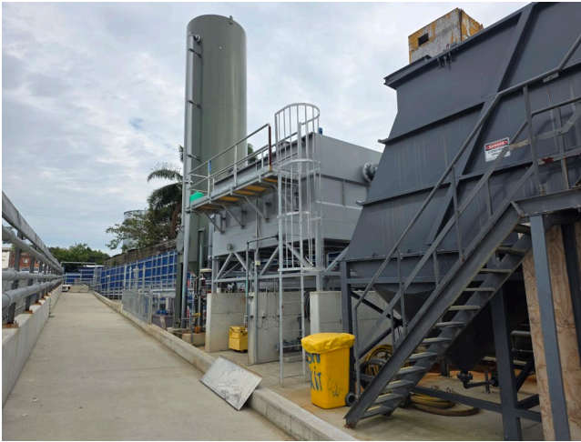
Figure 1.5 Water treatment plant recommissioned (Burwood North).
