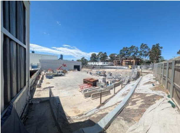
Figure 2.5 – Westmead (Surface level – Pad1): TBM demobilisation scope completed. Housekeeping /clean-up of Pad 1 commenced.
