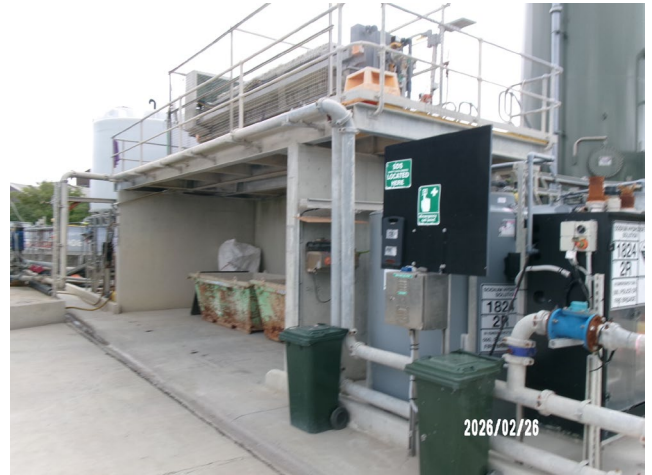
Figure 1.2 Ongoing operation of the water treatment plant at the Bays (The Bays).
