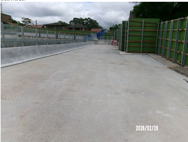
Figure 1.3 Eastern Shaft – Hardstand areas free of dirt and debris at the East Shaft (Five Dock).
