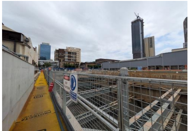
Figure 2.2 - Parramatta Western Station Box: Misters in operation for dust suppression on Western end.
