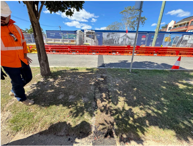
Figure 4.1 Road crossing outside 2 Second Ave was completed without the need for rock hammering. Trench backfill and temporary restoration with hotmix across the front of 2 Second Ave.
