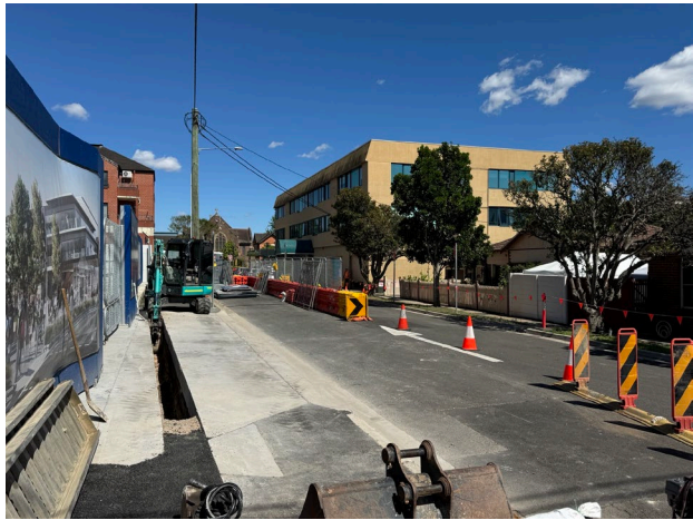
Figure 4.2 Spoil excavated and straight onto truck, without stockpiling onsite. No spoil stockpiling to occur at Second Ave MAF.
