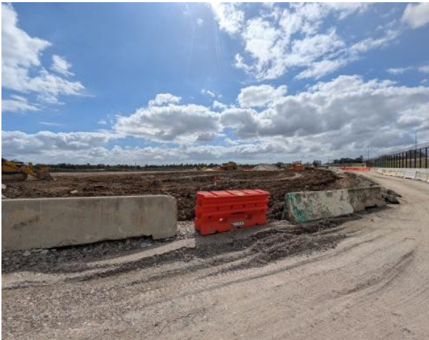
Figure 2.9 – Clyde MSF (West): Backfilling of previous crib and site office area ongoing.
