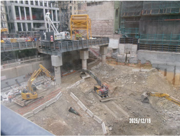
Figure 3.3 Hunter St West: Ongoing excavation of the shaft. Anchor installation under Hunter Street.
