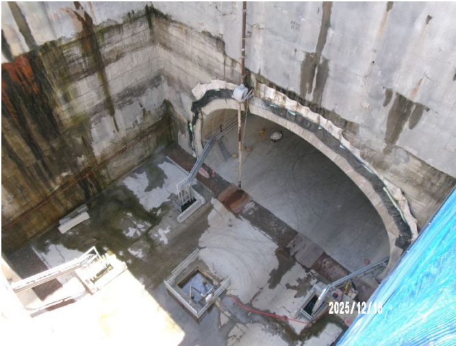
Figure 1.3 Eastern Shaft – No activities sighted. Automatic water management system operating at the base of the East Shaft (Five Dock).
