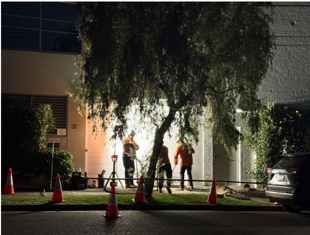
Figure 5.1 Worksite established on Waratah St, outside Focus Care building. Businesses (Focus Care and C3 Education) not operating during the works. Alternate Accommodation provided to residents.
