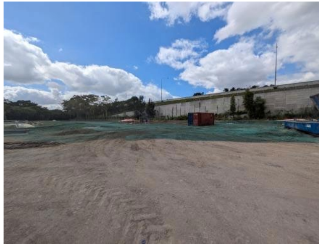
Figure 2.10 –Clyde MSF (West): Application of soil binder on exposed surfaces in preparation for Christmas shutdown.
