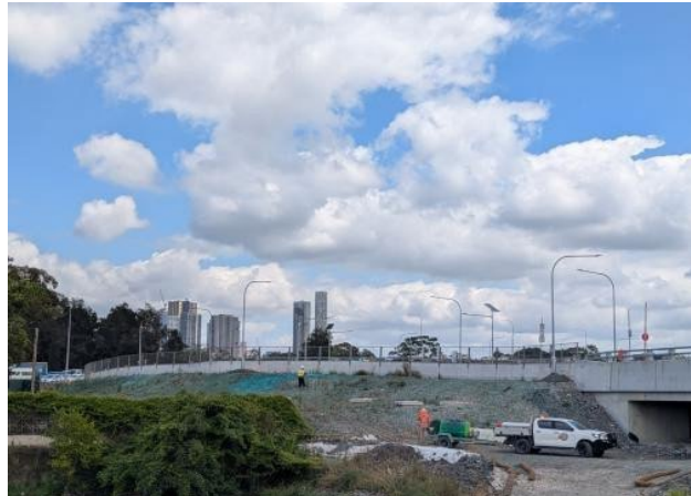
Figure 2.8 – Clyde MSF (West) – Application of soil binder on embankments commenced in preparation for Christmas shutdown.
