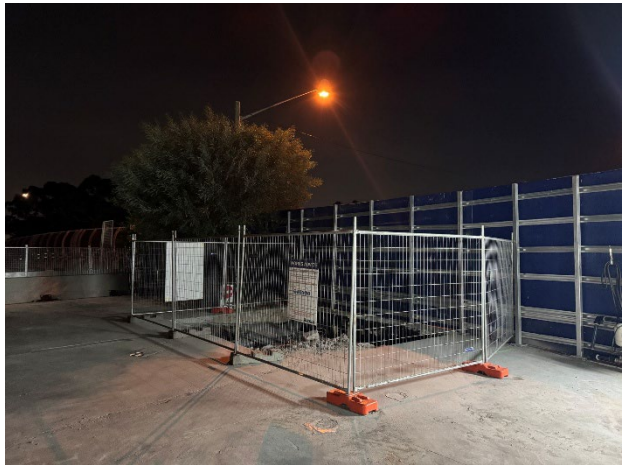
Figure 5.2 Hoarding modification undertaken 6th December across the front of the electrical kiosk location, offering a noise barrier for most of the upcoming works associated with siting the kiosk.
