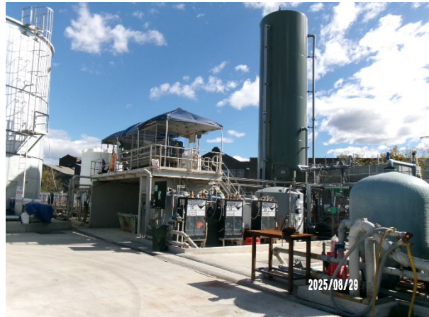
Figure 1.2 The water treatment plant operating at the Bays (The Bays).
