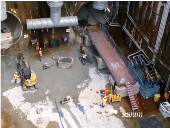
Figure 1.1 Station Box (The Bays). Services pits in the base of the station box were being moved.
