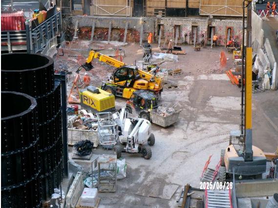
Figure 3.1 Hunter Street East: Former Acoustic Shed area. Wall support along the O'Connell Street boundary.
