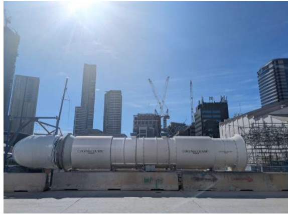
Figure 2.2- Parramatta Site: Ventilation fan installed and operational.
