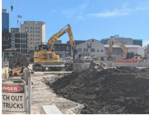
Figure 2.4 – Parramatta Site: Zone 9b - concrete slab removal, with misting canon operational to manage dust.
