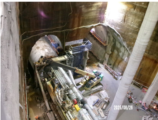
Figure 3.5 Pyrmont East: TBM Ruby traversed into the nozzle. Works in the nozzles to prepare for TBM re-launch.
