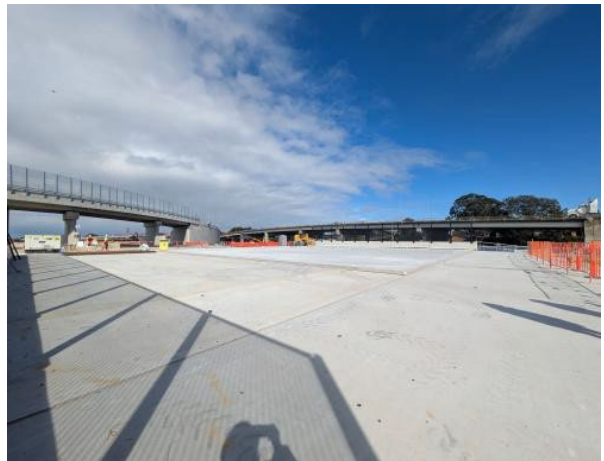
Figure 2.12 – Clyde MSF Site: Flood Relief Bridge with secondary slab poured to accommodate workshops being relocated from Clyde Dive.
