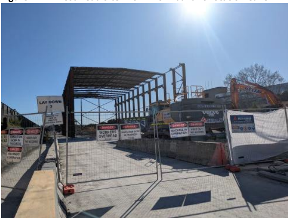
Figure 2.9 – Clyde Dive Site: Acoustic Shed demolition works – all panels removed; with steel frame to be removed.
