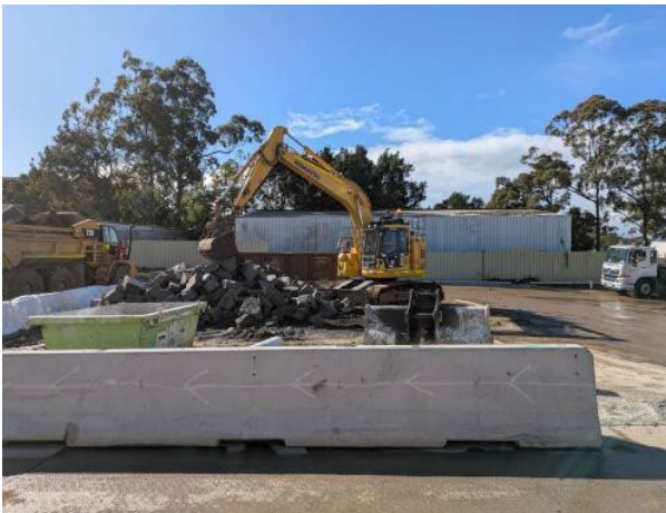
Figure 2.11 – Clyde Dive: Concrete stockpile from haul road removal works along eastern boundary.
