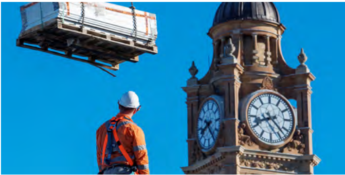
Image: Solar panel installation at Central Station contributing to carbon emissions reduction.
