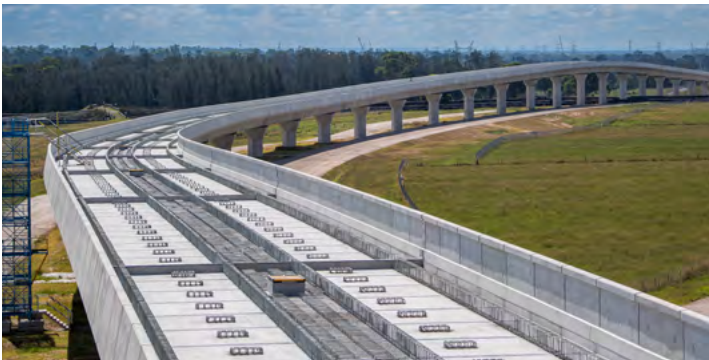
Image: Elevated viaduct between Orchard Hills and Luddenham.
