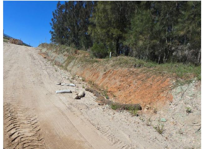
Luddenham to M12 – ESC required reinstating.
