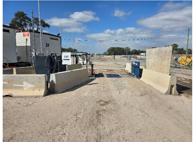
OHE – Landsdowne Rd exit wheel wash was not operating during the inspection. Tracking was maintained via a street sweeper.
