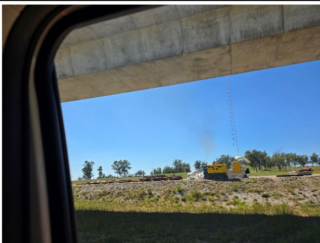
Water Pipeline to Luddenham Station –Noted a generator had smoke emission. PLM undertook maintenance on the generator.
