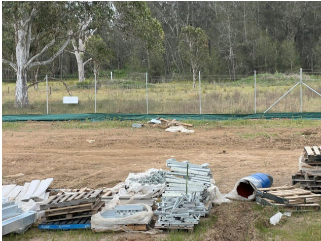
Patons Ln to water pipeline – Removal of work materials and litter from ancillary facility demobilisation was required.
