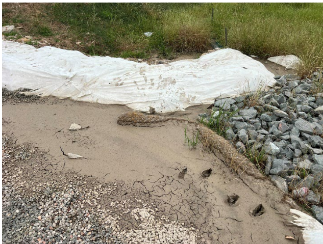
SMF – Maintenance of ESC was required post-storm event.
