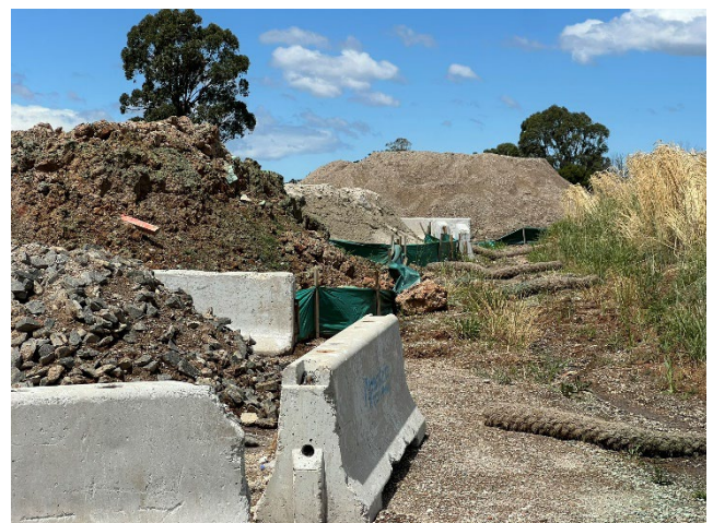
BSF – Sediment fences required reinstating post storm event.
