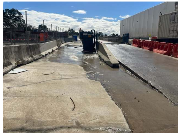
Photo 24: The wheel wash was being emptied with dirty water discharged to the sediment basin
