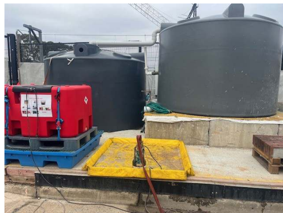
Photo 3: Water treatment tanks discharged to cess via permit or reused. Fuel cell.
