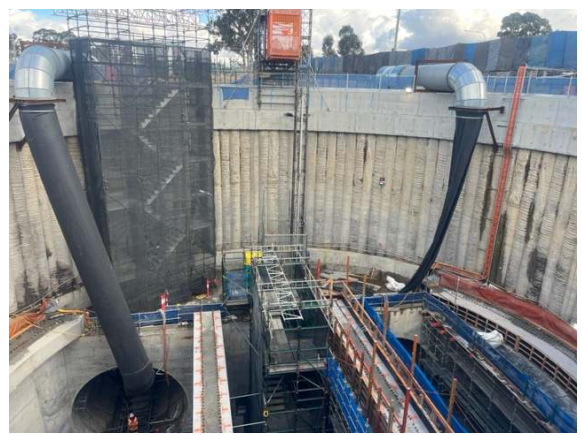
Photo 53: Shaft for deliveries into tunnel & ventilation system
