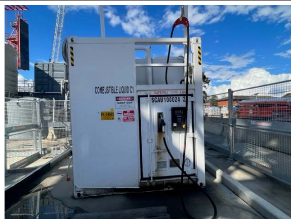
Photo 60: Diesel storage tank – self-bunded and compliant GHS signage
