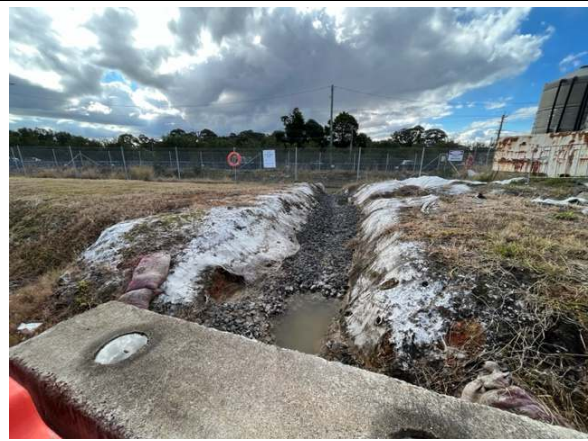
Photo 50: Holding basin associated with Water treatment plant
