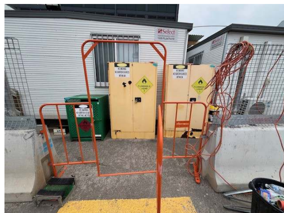
Photo 5: Compliant hazardous chemical storage.
