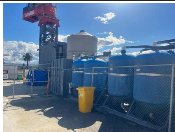
Photo 59: Water treatment plant operational with discharge to sewer under TWA
