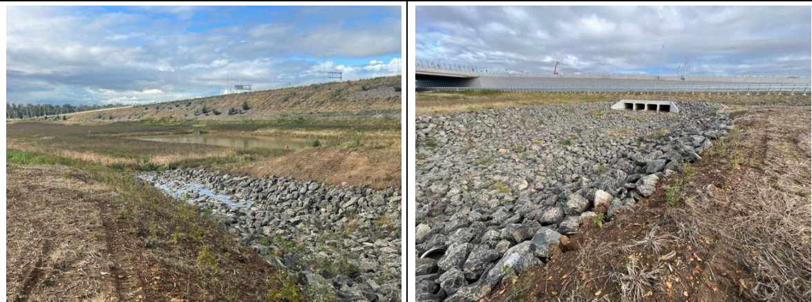
Photos 3 & 4: Sydney Water swale discharging to bioretention basin and Sydney Metro basin. Dewatering is not required from the Sydney Metro basin.
