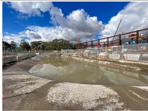
Photo 23: Sediment / holding basin for site runoff, including from wheel wash. Water is reused for dust suppression or transported to the WTP at Claremont Meadows
