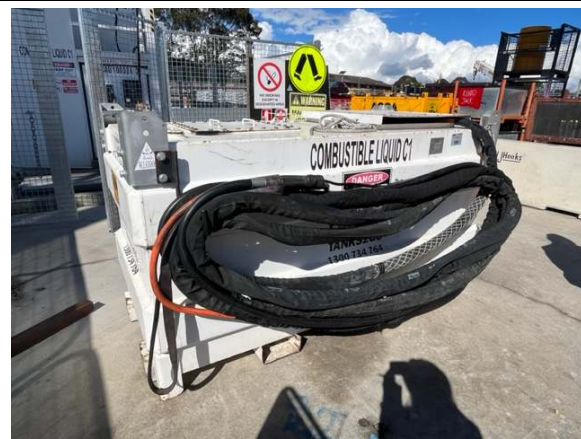
Photo 61: Diesel fuel cell - self-bunded and compliant GHS signage
