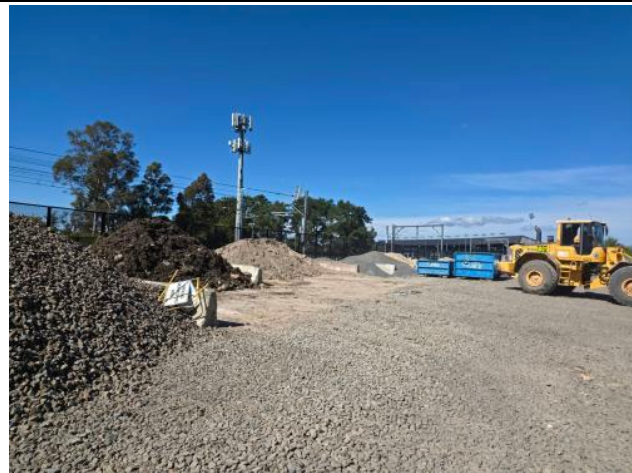
Figure 3 – Belmore Triangle. JHLOR reports that access into the rail corridor from Belmore triangle hi-rail pad is currently not being used. Various material stockpiles were observed within the laydown area including ballast for recycling, restricted general solid waste and asbestos containing material.
