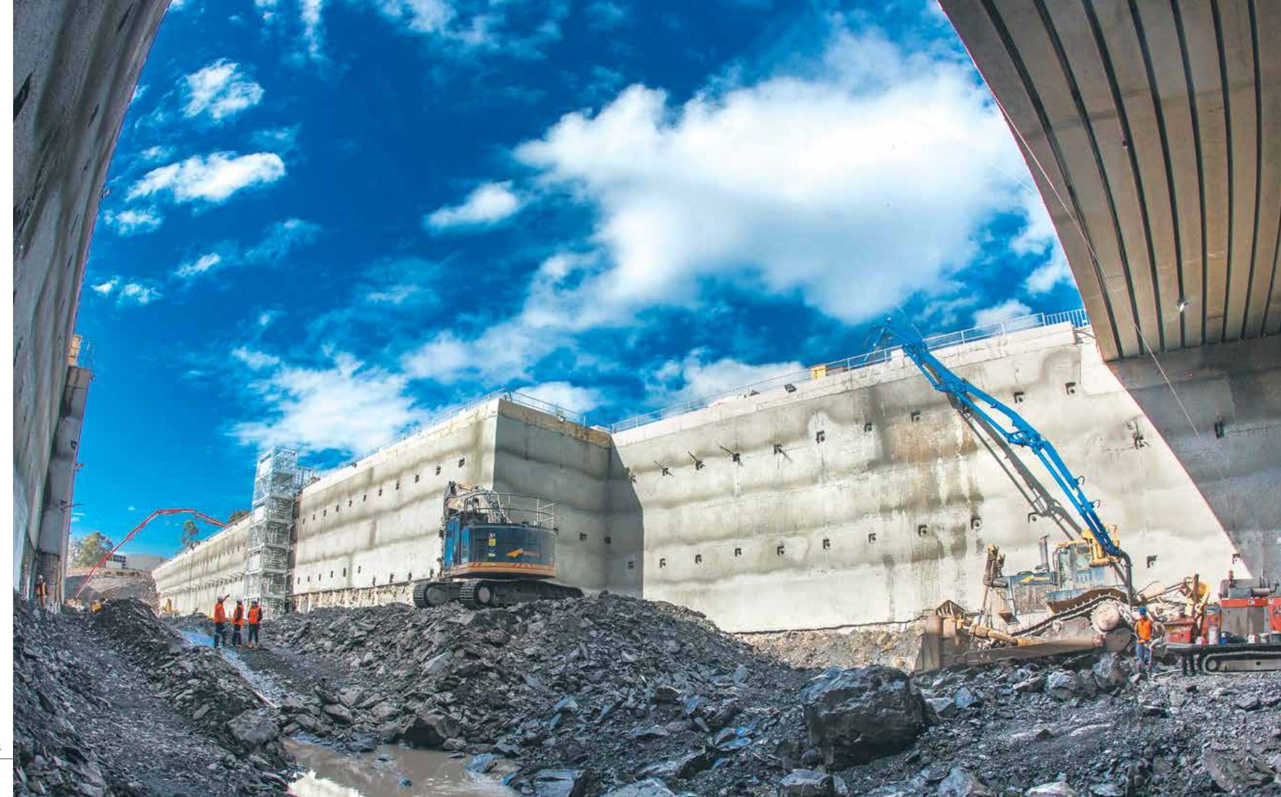
Norwest Station with the temporary bridge at top right of picture, July 2014
