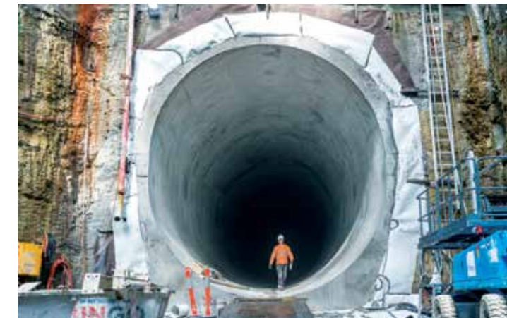
Two 300m long tunnels linking the new twin tunnels to the existing railway tunnels between Epping and Chatswood were completed in mid-2015
