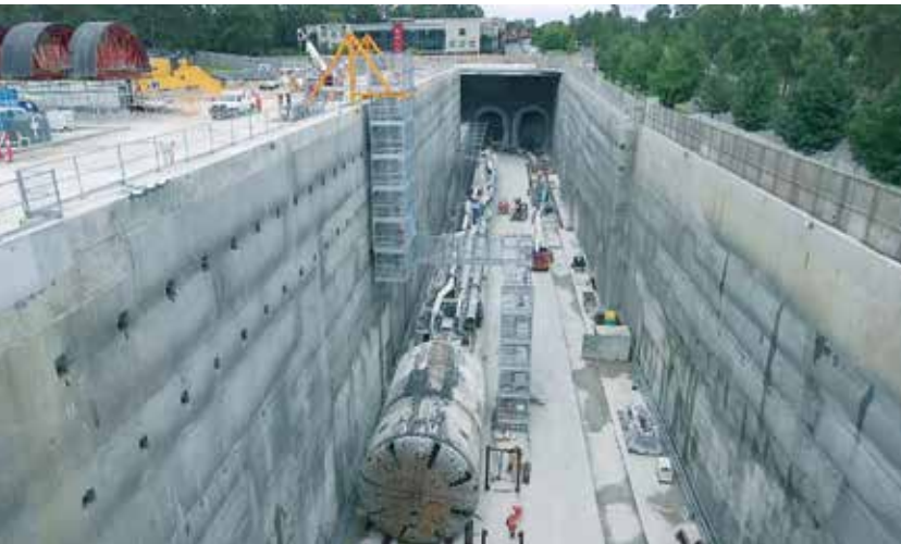
Following the first break-through, TBM1 Elizabeth traverses the Norwest Station site, February 2015
