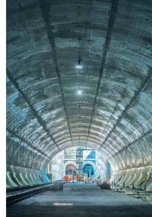
View from the crossover cavern to the future Castle Hill Station site, October 2015
