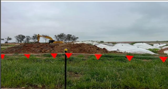
Elizabeth Drive compound – ACM was being loaded out and taken to PS105
