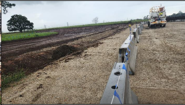
SMF – Topsoil stripping for light vehicle carpark, with tree protection zones were maintained.
