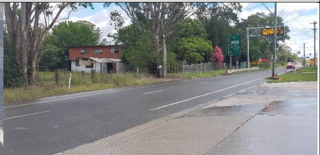
Kent road view north at site access – Negligible tracking with only historical veneer noted. Road in good condition.
