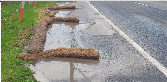
Orchard Hills Kent road view south at site access – Erosion and sediment controls well implemented .
