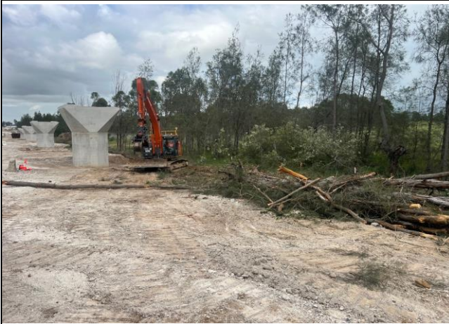
Defence land – Additional clearing is required to accommodate the width of the viaduct
