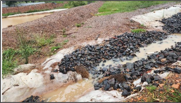
ORH –Swale to the storage dam required additional erosion controls and re-pinning of geofabric.
