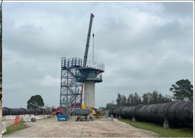
Warragamba Pipelines – Works have commenced between the pipelines, vibration monitoring is being undertaken
