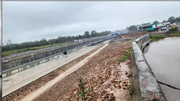
ORH – Scouring of the northern embankment, work to extend the apron had commenced and haul road over the swale was improved. Installation of long-term erosion and sediment controls remained an outstanding action.
