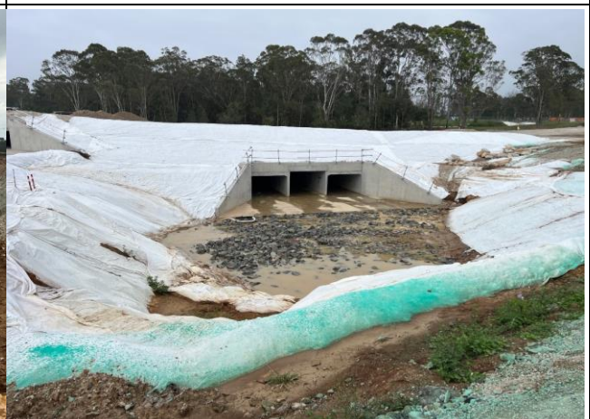
Unnamed tributary – Scours have occurred at the unnamed tributary culvert. It is noted that the project team used their system to detect and commence rectification works
