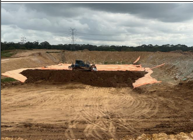
PS105 – ACM is being deposited at PS105 in accordance with the RAP
