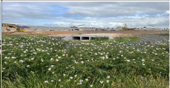
Elizabeth Drive compound – weeds are present onsite, however spraying has commenced
