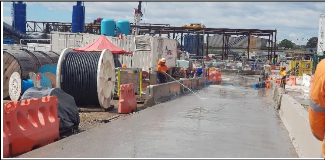
Orchard Hills view south – Internal haul road to exit apron free of tracking.
