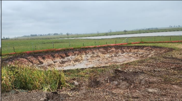
LUD –Temporary catchment pond adjacent to piling works. PLM indicate that this would be utilised for dust suppression and pumped out regularly to prevent overflow.
