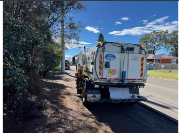
Hobart St – A street sweeper is onsite and follows the existing spoil truck
