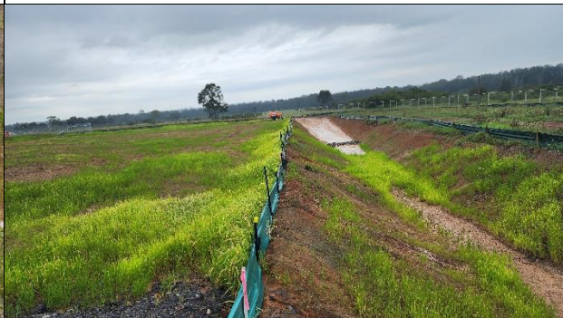
AEC – Realignment of the boundary clean water swale with pump to sediment basin.
