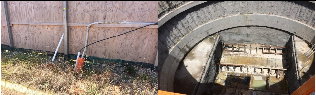
Bringelly northern boundary – Erosion and sediment controls require refreshing.
