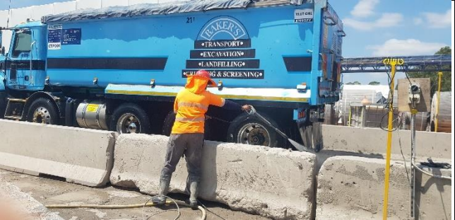
Orchard Hills – Tunnel spoil haulage truck with project signage at manual wheel wash.
