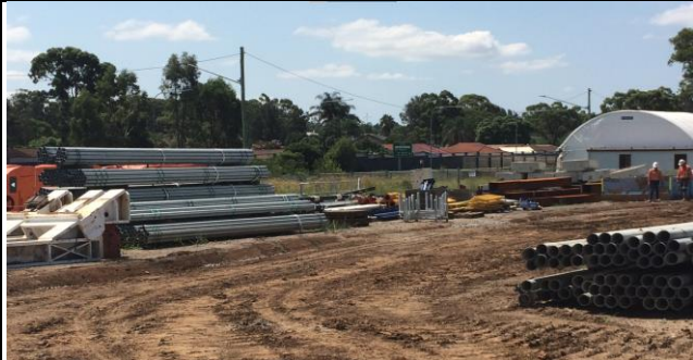
Claremont Meadows western areas – Implementation of ESCP reviewed by Soil Conservationist underway.
