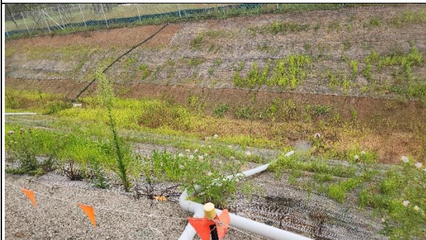
AEC – Stabilisation of the stormwater discharge to the clean water diversion to be completed
