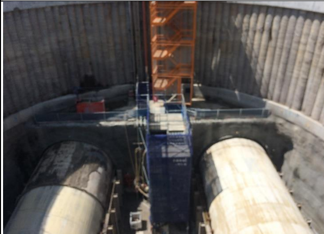
Claremont Meadows shaft view north – TBM Catherine tunnel (right), and TBM Marlene finalising traverse (left) – note TBM head shield tail (dark areas).
