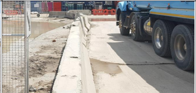
Orchard Hills view west – Internal spoil haul road repaired. Note condition of road/ HV tyres prior to wheel wash.
