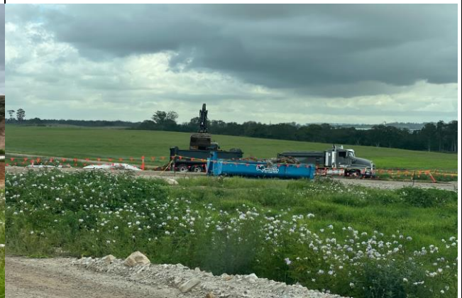
Elizabeth Drive compound – ACM is being loaded out to PS105, controls were in place to reduce accidental spillage
