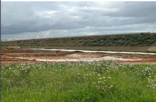
SCAW – M12 interface – Water is released from the M12 project without warning to SCAW. A notification from M12 needs to be made to ensure SCAW has sufficient capacity to accept the water
