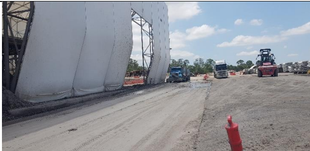
Orchard Hills view north – Internal spoil haul road repaired and in significantly improved condition.
