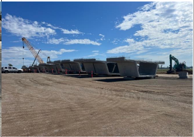
Luddenham South - Segments have been stacked to accurately facilitate the sequence and access by the crane
