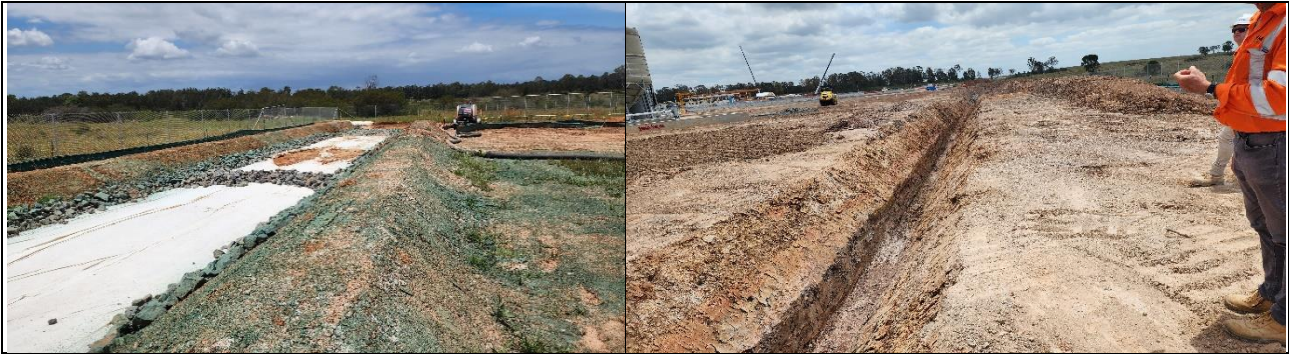
AEC – Discharge swale from water treatment dam. PLM noted that geofabric required repining.
