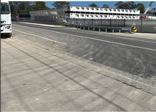
Lansdowne Road - Minor mounts of dirt have been tracked out of the site, however a street sweeper has been stationed there to clean the road
