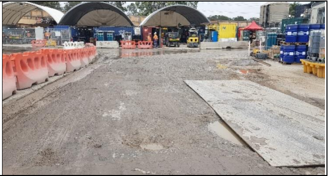
Orchard Hills view west: Internal spoil haul road in poor condition and requiring repairs.
