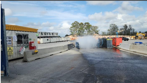
STM – Barriers installed to direct vehicles through the wheel wash and site compound installation
