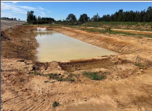
Cosgroves Creek – The sediment basin has been constructed as per ESCPs however requires a spillway
