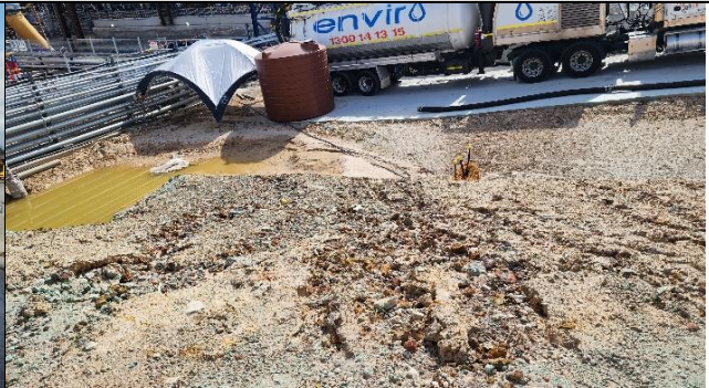
ORH – Scouring of the northern embankment. PLM agreed to install long term erosion and sediment controls
