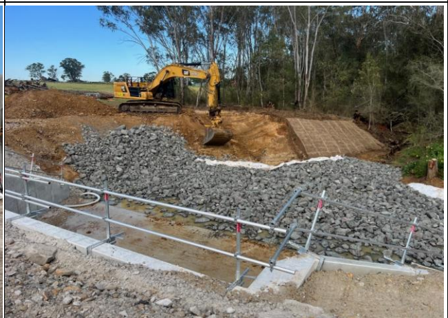
Unnamed tributary - A clean water inlet is being constructed into the culvert
