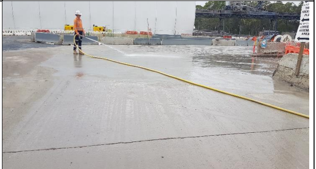
Orchard Hills exit: Greater frequency of washdown needed to minimise tracking onto Kent Rd.
