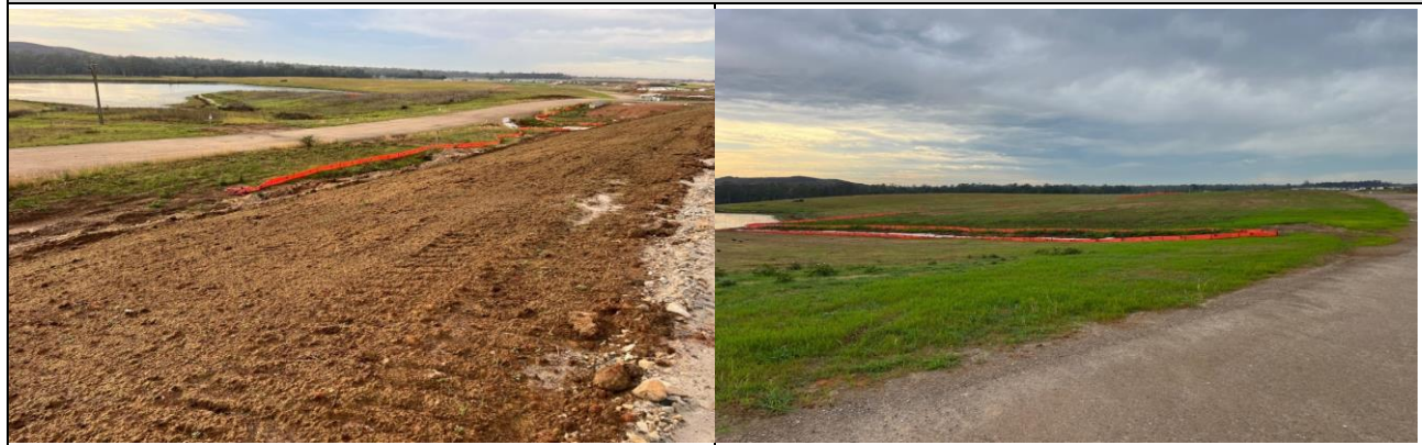
M12 Bridge - Topsoil and hydromulch has been applied to batters at M12 bridge, providing a stabilised surface Elizabeth Drive Haul Road - Regrowth of hydromulched areas has been successful following recent wet weather
