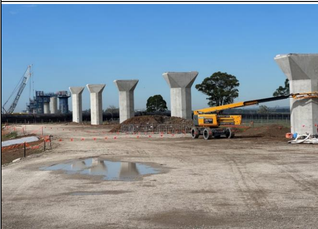
Defence - Works are progressing well near the Warragamba pipelines. Vibration monitoring has been compliant with the Water NSW requirements
