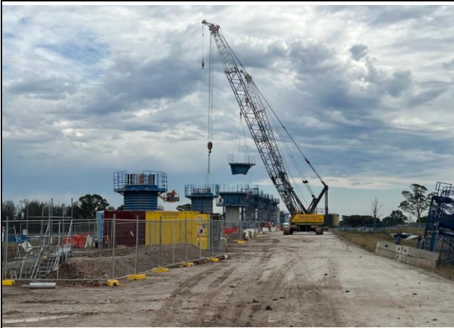
Luddenham North - Forms are being installed ready for concrete pours in the new year
