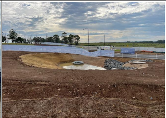
Luddenham North - The ERSED controls on the new Celestino access road are well installed and look to be effective
