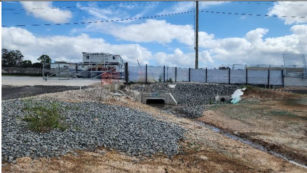
ORH – Noted scouring of swale. PLM agreed to place more rock to reduce scouring.
