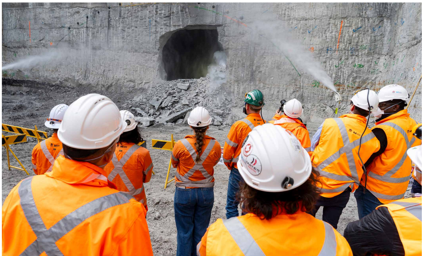
Image: A roadheader breaks through at Five Dock with excavation work continuing at the Station site.
