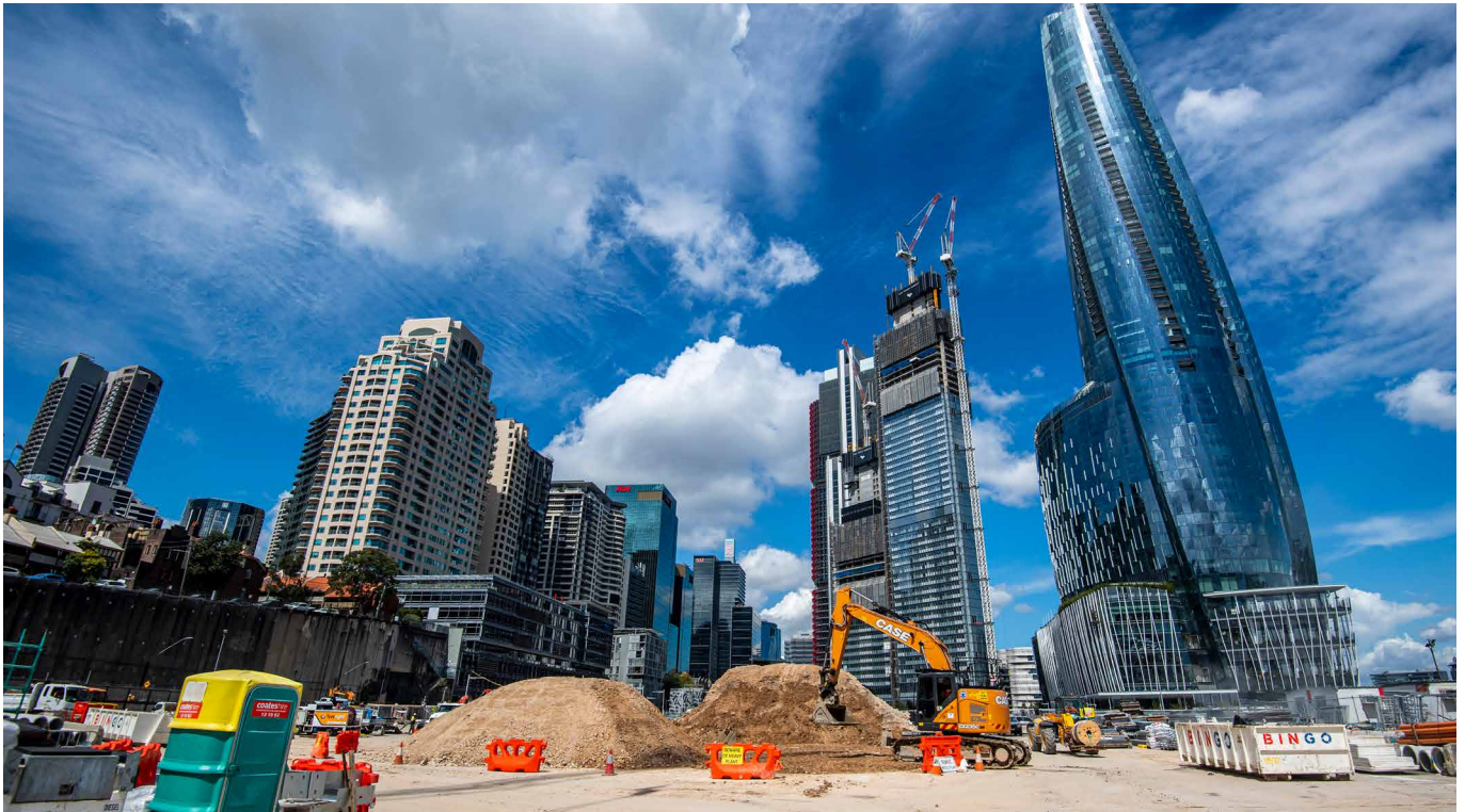
Image: Spoil from other sites being delivered to the Barangaroo site to be used for the new Hickson Road construction.
