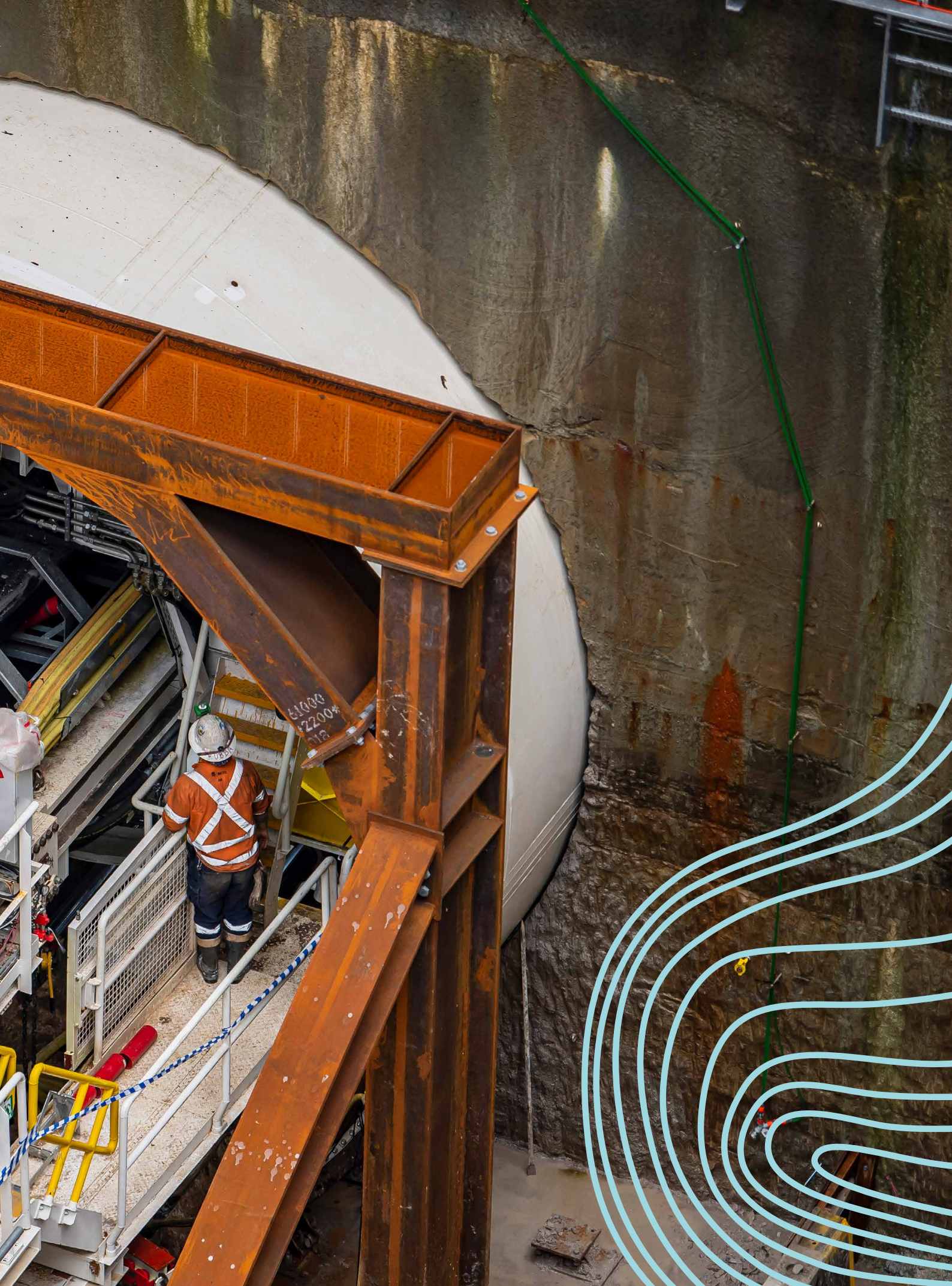
Image: Tunnel Boring Machine Daphne continues its early progress at Sydney Metro's The Bays station site.
