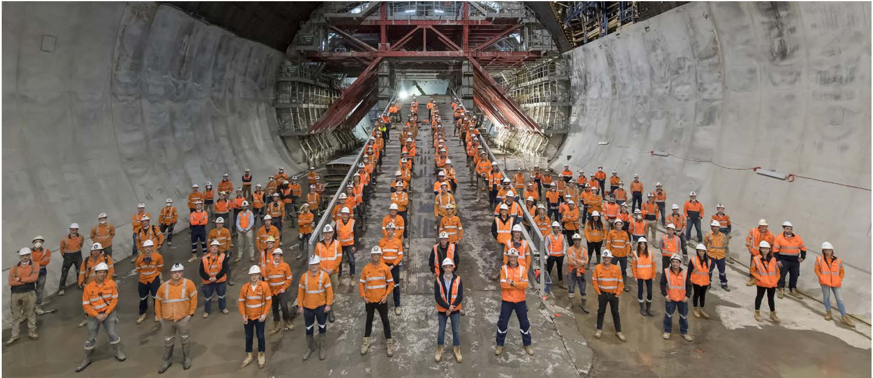
A team of workers about 31 metres underground at the Sydney Metro City & Southwest Victoria Cross Station, in the heart of the North Sydney business district.
