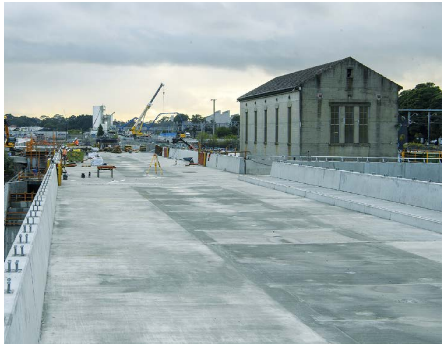
Construction of the new aqueduct over the existing heritage-listed Sydenham Pit, while retaining the existing heritage listed pump station.
