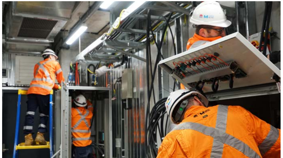
Workers installing high voltage control panels in one of the 26 equipment rooms within Central Station.
