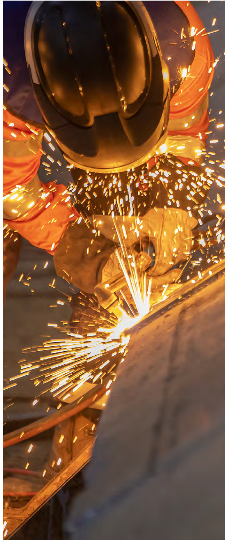
Work continues on the metro railway tunnels under Sydney Harbour, 30 metres below ground from Barangaroo.
