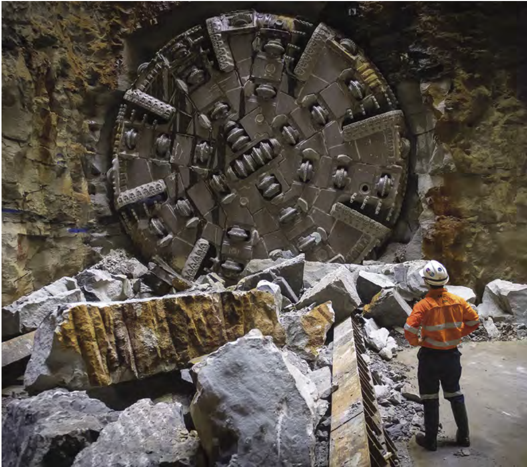
TBM 3 Wendy, dug a 6.2-kilometre tunnel to the edge of Sydney Harbour, on the City & Southwest project.
