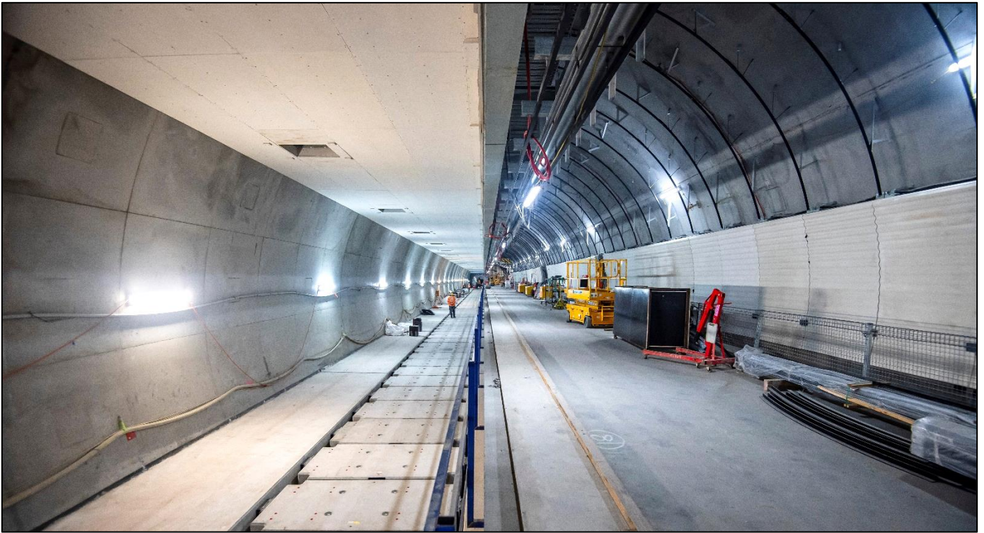
Pitt Street Station underground cavern where work is taking place to fit out the platforms and tunnels.
