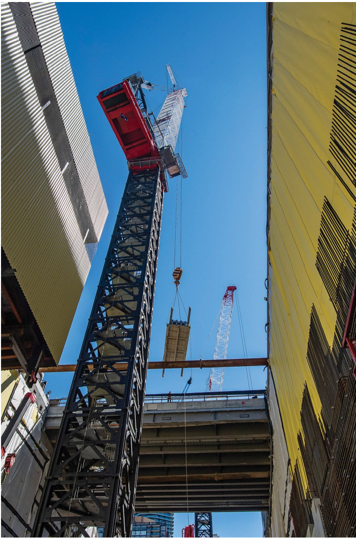
Muscles, the tower crane at Crows Nest Station site. The tower crane was named by Kelly's Place, a local child care centre.
