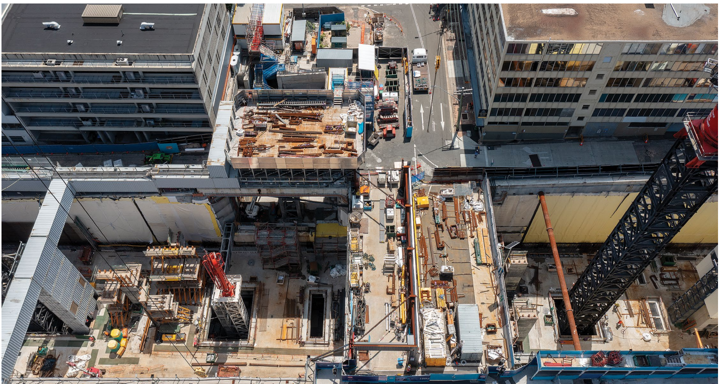
Aerial image of Clarke Lane and Hume Street with station build below.
