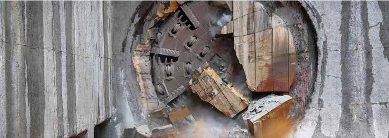
Tunnel boring machine Nancy breaking through at Barangaroo metro station on Sydney Metro, City & Southwest.
