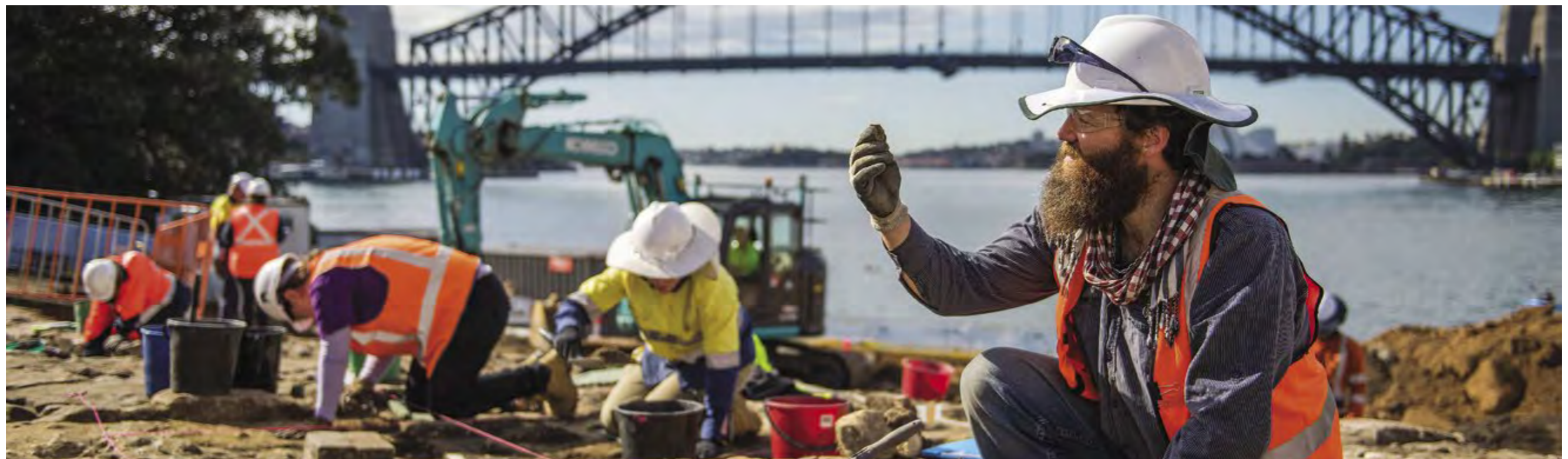
Uncovering heritage artefacts at Blues Point on the Sydney Metro City & Southwest project.
