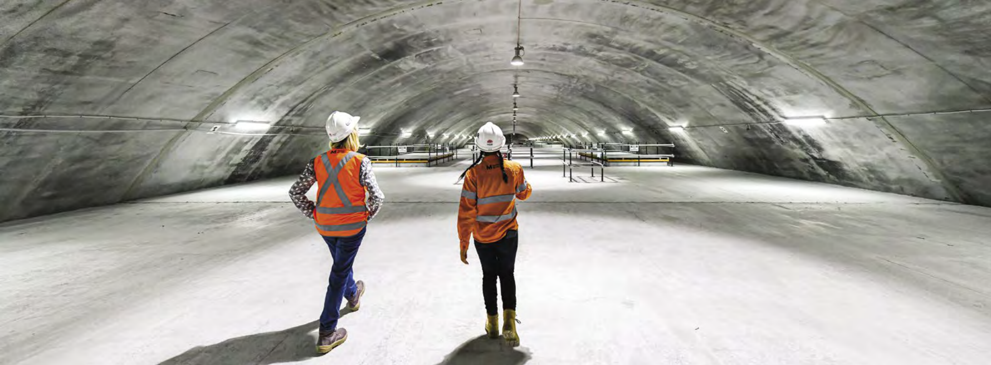
Cavern view of progress works on the Sydney Metro City & Southwest project.
