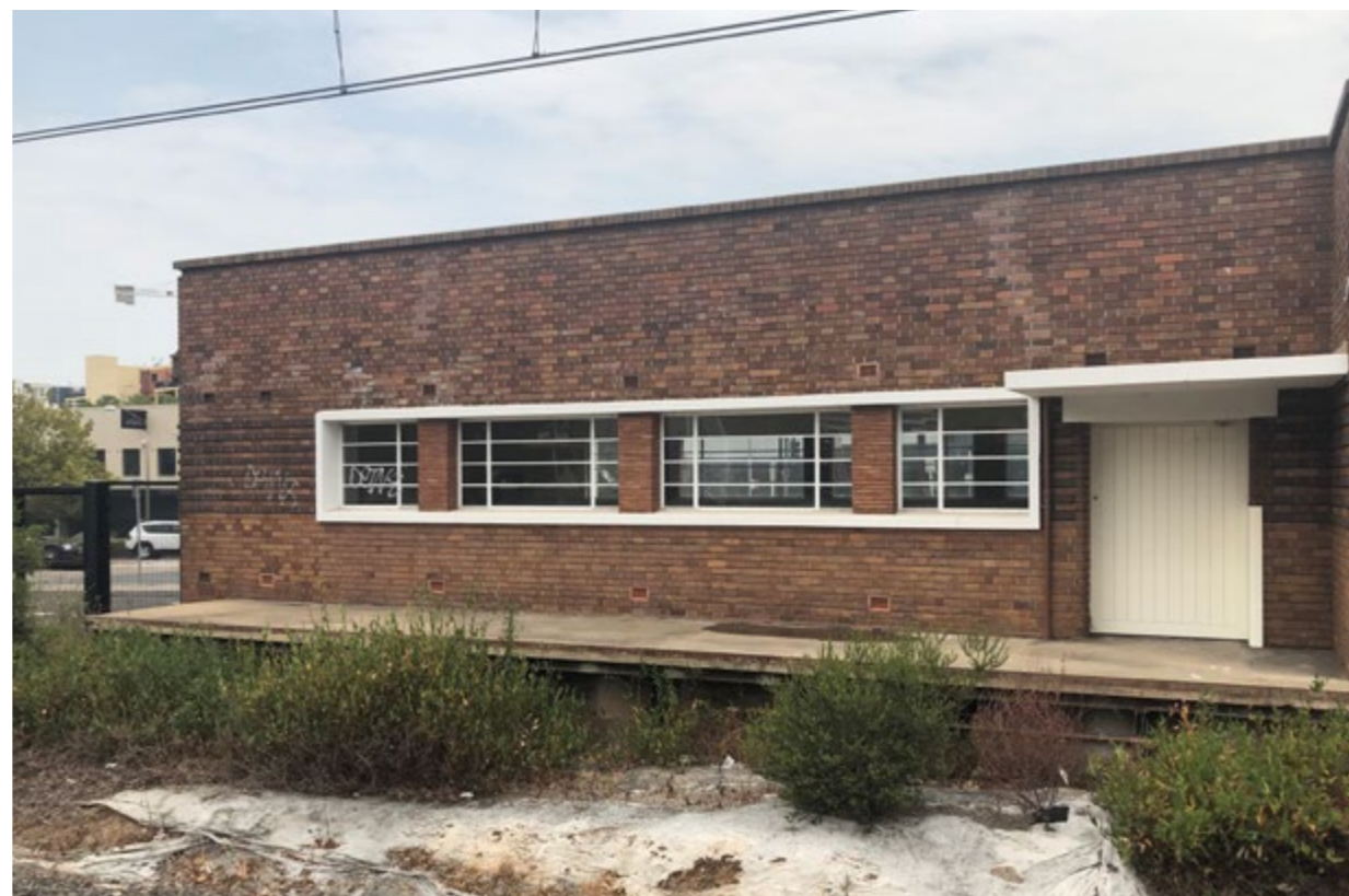
Figure 4.13 Parcels Office present day condition - as viewed from Bankstown Station platform
