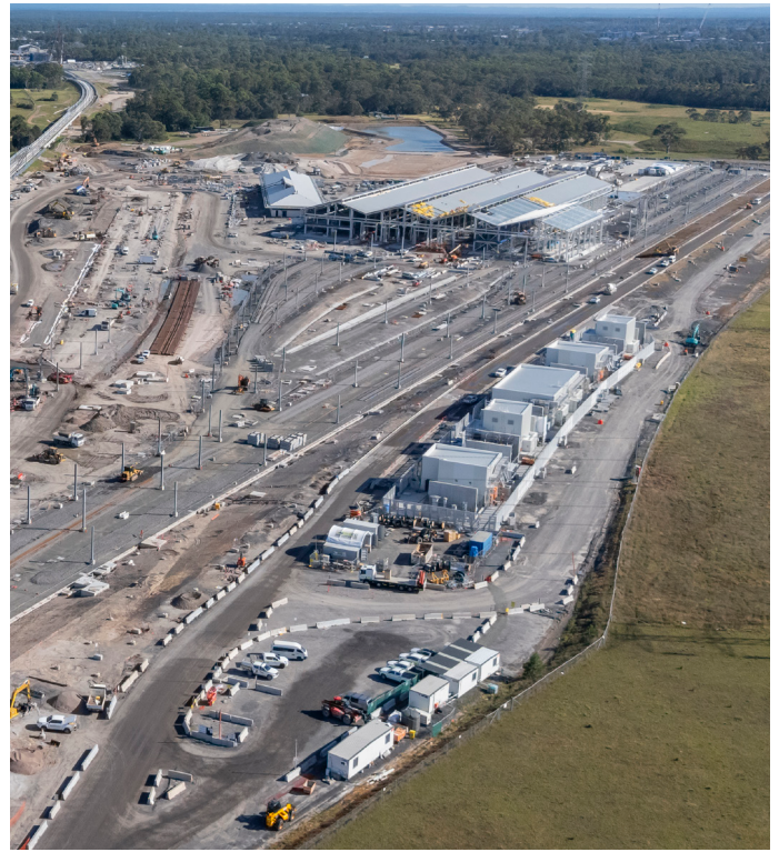
The Stabling and Maintenance Facility has received 132kV bulk power supply from the Endeavour Energy grid.
