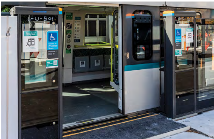
Testing platform screen doors across Southwest stations.
