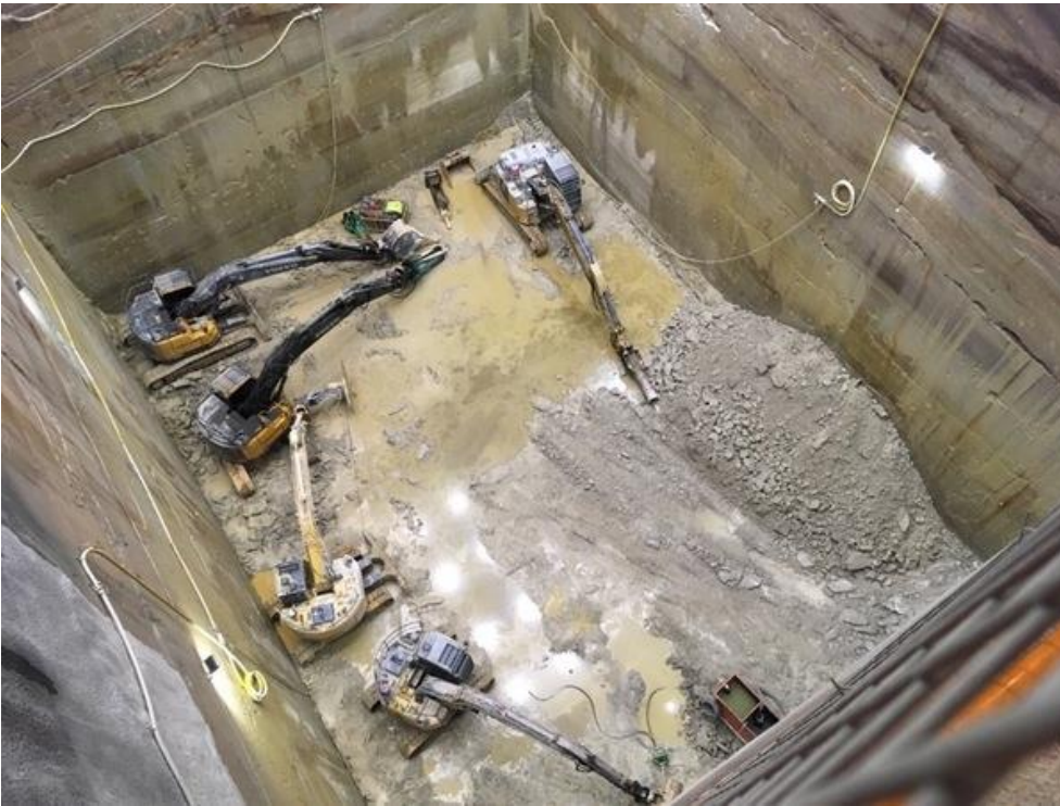
Excavation of the new lift access shaft is currently approximately 37 metres deep
