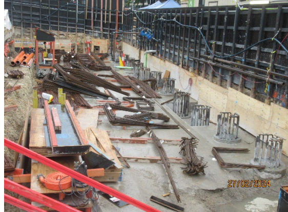
Figure 3.2 Pyrmont East: Pile caps broken back on the piles along Union Street boundary
