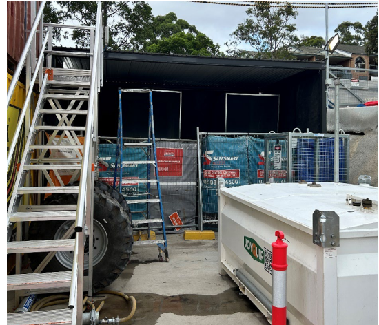
Figure 2.2: Westmead site – Air compressors with noise attenuation
