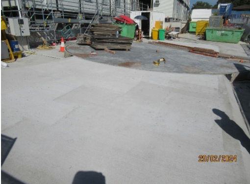
Figure 1 3 Truck turntable installed in the south entry of the Western Shaft (Five Dock).
