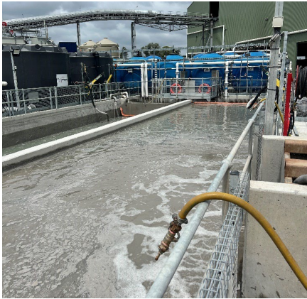
Figure 2.7: Rosehill Site – Water Treatment Plant operation
