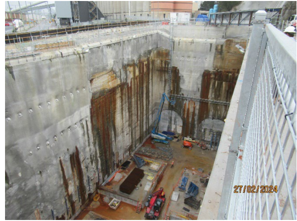
Figure 3.8 The Bays: TBM launch support structures being constructed in the base of the station box. Niches concreted.
