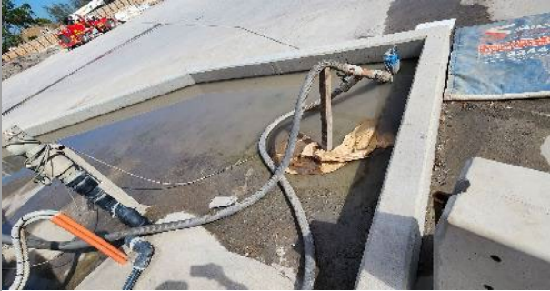
Photos 17-18: bunded areas with stormwater ponding
