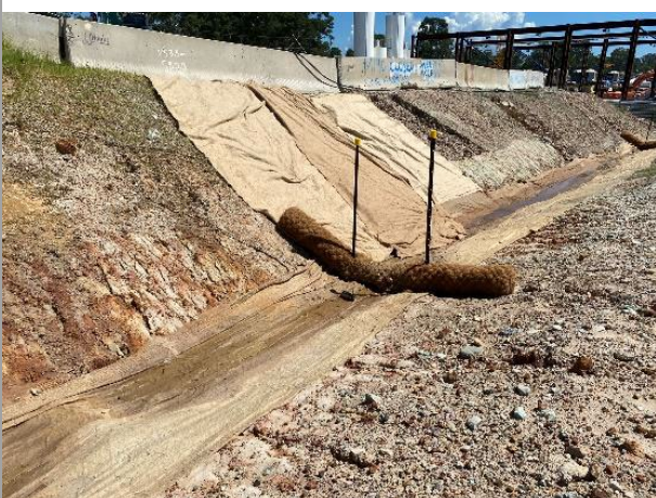
Photos 28-29: Erosion control devices in place
