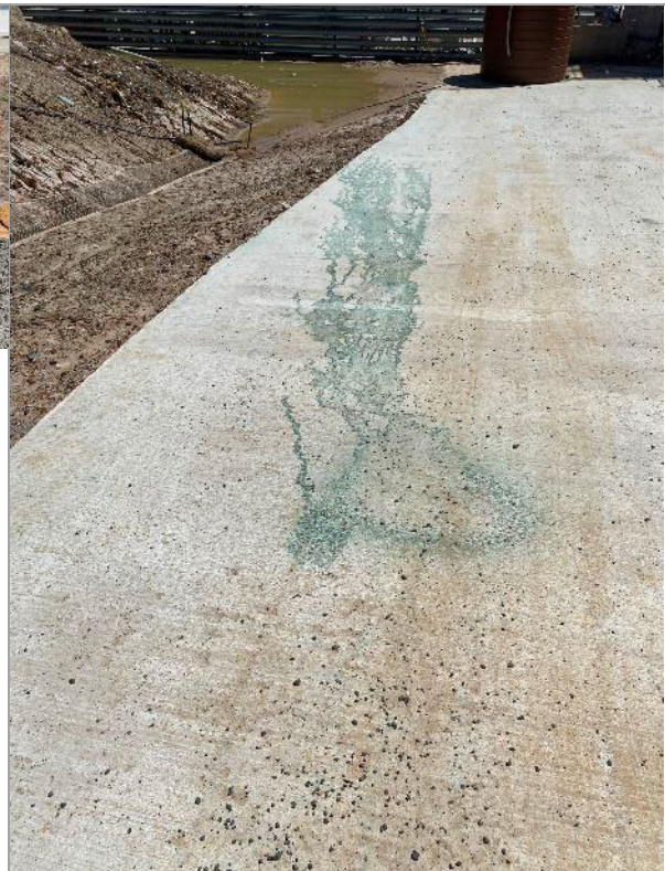
Photo 30: Random unconfirmed colouring on pavement (presumed to be dust control chemical)
