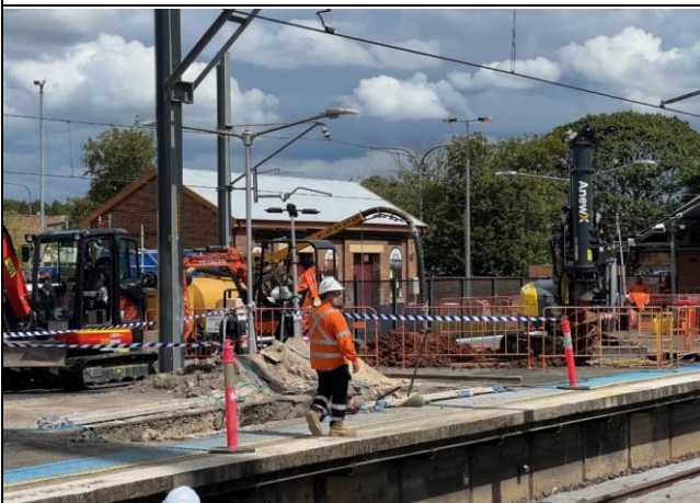
Platform - A vac truck was used for NDD tasks, minimising turbid water spillage risk.
