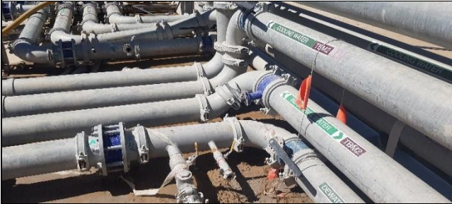
Orchard Hills south – CPBG to endeavour to rectify potable water leak during TBM Easter maintenance.
