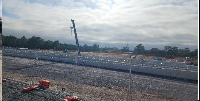
ORH –Reshaping of the western batter was ongoing. Topsoil stripping and reshaping for the concrete batch plant had commenced
