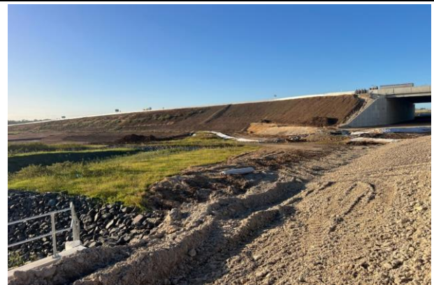
M12 Interface - Design options are ongoing within the CPB steering committee to resolve how M12 water will be handled
