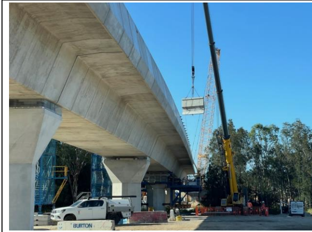
Cosgrove's Creek - Parapets are being installed along the viaduct over Cosgrove's Creek
