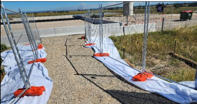
LUD –It was noted that additional erosion and sediment controls at the crossing of the swale were installed. PLM has engineered a solution to remove the bund and will install a shipping container bridge.
