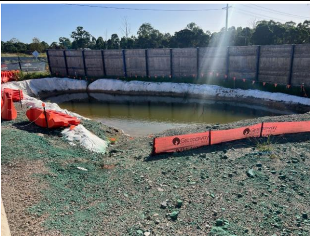
Lansdowne Rd - An existing sump is being used to retain water from inundating the neighbouring property
