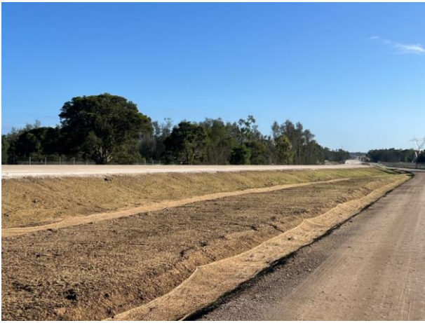
Defence - Drainage is nearing completion, with jute mat installed and spray grass germinating
