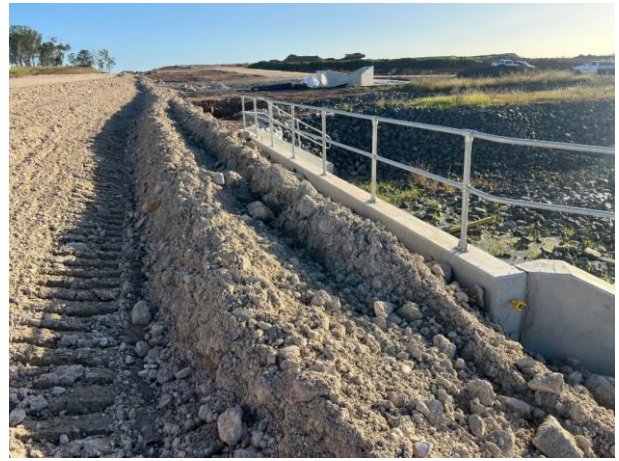
M12 Interface - The bund on top of the southern culvert is a good idea and will need to be monitored regularly
