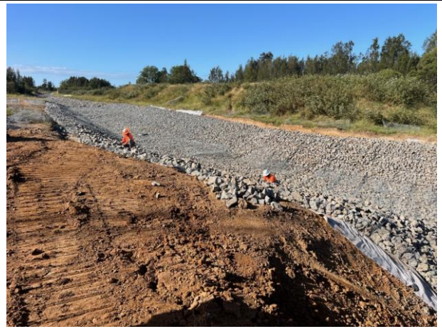
Cosgrove's Creek - The works in the rock mattress lined drain are ongoing
