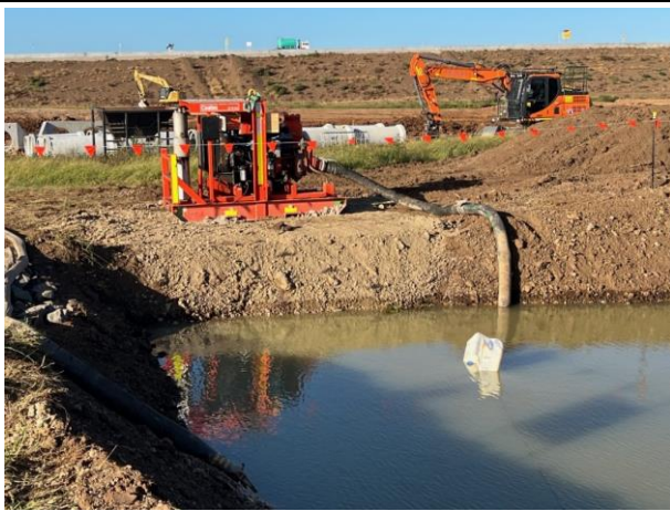
EDR Entrance - A new sediment basin has been established that can take the SCAW runoff while keeping the larger basin dry
