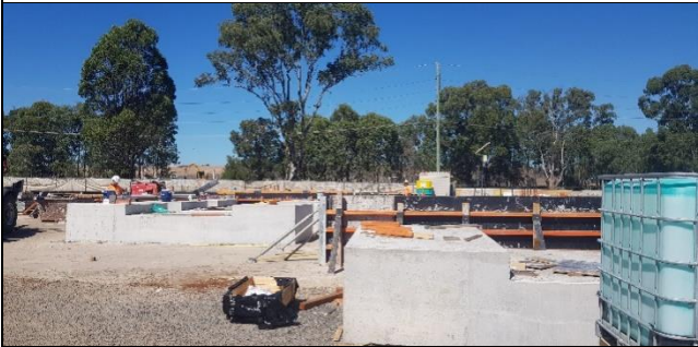
Claremont Meadows western areas – Pre-cast of TBM support blocks for St Marys TBM retrieval.
