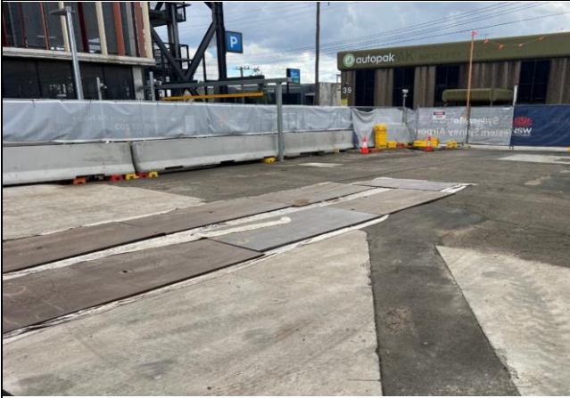
Compound - Temporary road plates have been placed over the cracked pavement to reduce mud tracking until the permanent solution is constructed.
