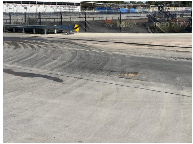
Lansdowne Rd - Minor dust levels have been tracked onto Lansdowne Rd, CPBUI to ensure a sweeper is available when required
