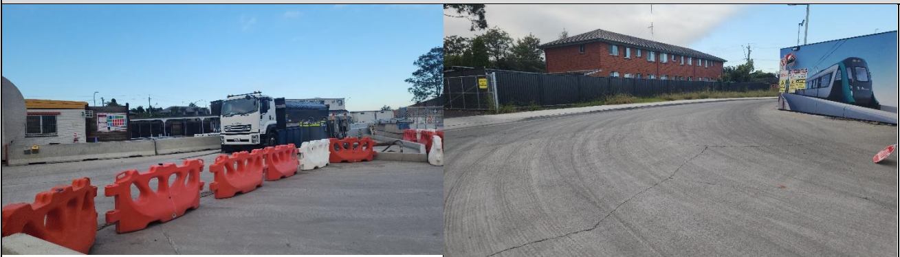
STM – Wheel wash was deactivated. PLM reactivated when raised as a site action by the ER.
