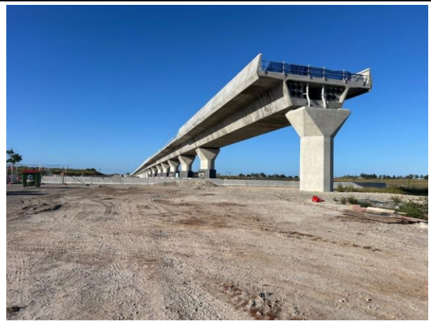
Luddenham North - The viaduct works are complete, until the last gantry establishment will complete the viaduct
