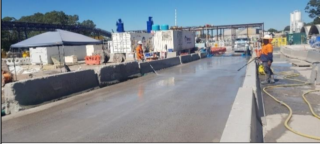
Orchard Hills view south – Internal haul road to exit apron in good condition.
