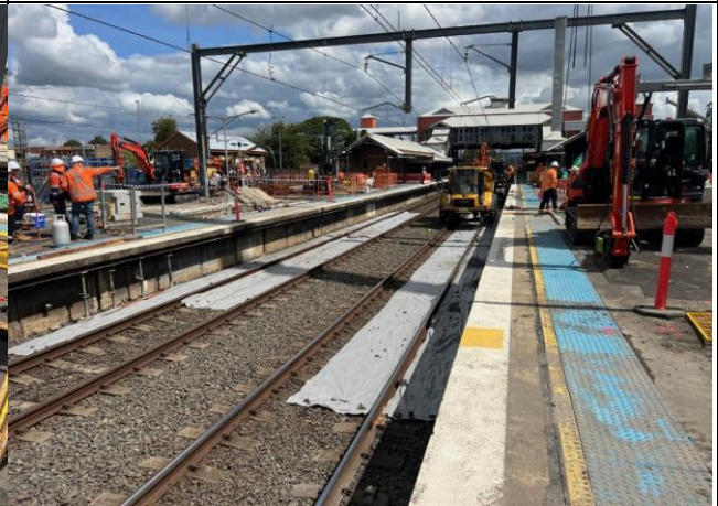
Platform - Geofabric is placed on the ballast to capture any material spillage and reduce the risk of ballast becoming fouled.
