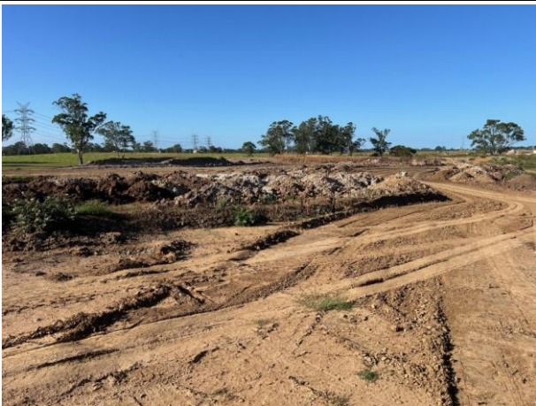
PS105 - Unsuitable material is being stockpiled on top of the containment cell at PS105
