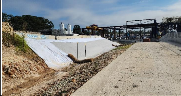
ORH –Erosion and sediment controls installed on northern batter. Installation of controls was ongoing
