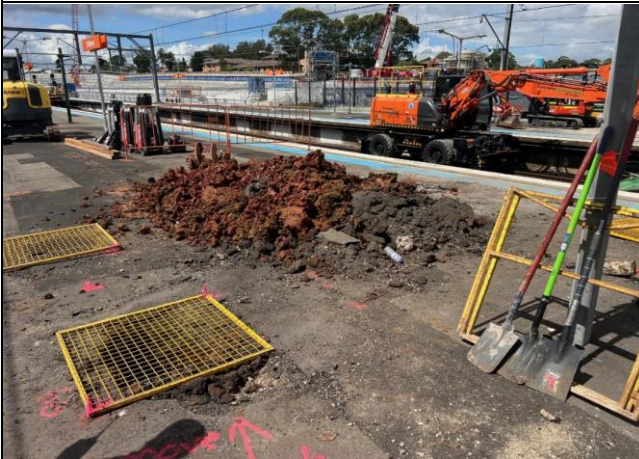
Platform - Pile spoil is temporarily stored on the platform prior to being loaded out.
