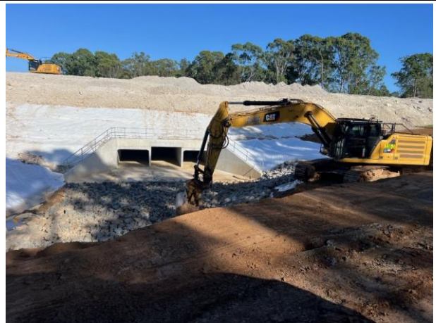
Unnamed Tributary - Works continue to finalise the scour rock at the culvert
