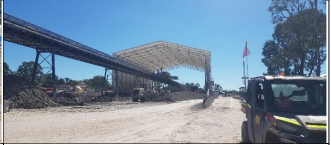
Orchard Hills view north – Tunnel spoil storage area continues to be well managed.
