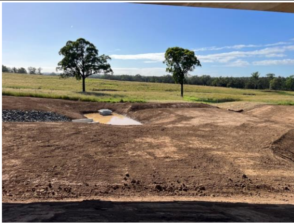
Luddenham South - Small sumps are utilised across the site to minimise construction water runoff
