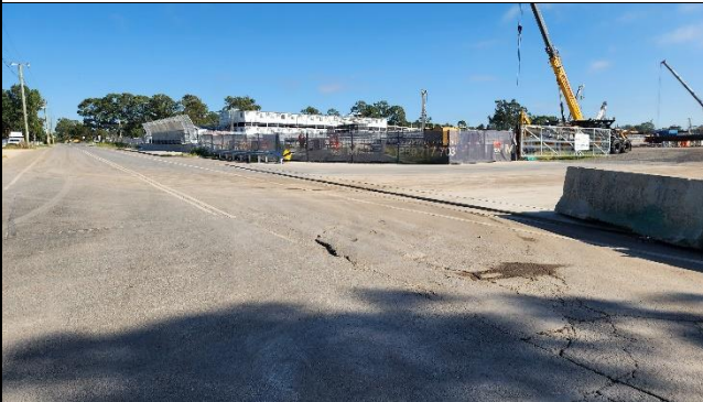
ORH –Sediment tracking from the concrete batch plant earthworks
