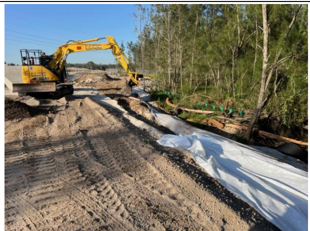
Defence - The upstream side of the unnamed creek is in the process of having its ERSED controls refreshed
