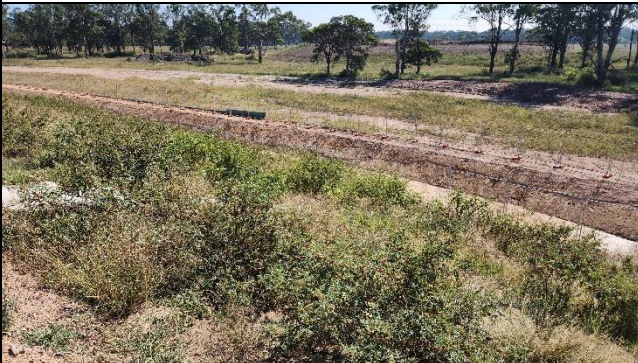
SMF – Construction of a water sump had been completed for storage of additional water for reuse onsite.
