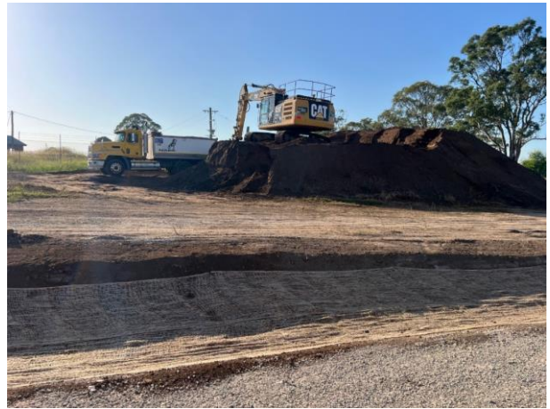
Defence - Topsoil is being loaded out from the southern Defence site, dust generation was minimal
