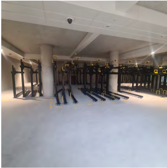
WL ISD: Bike storage racks installed.
