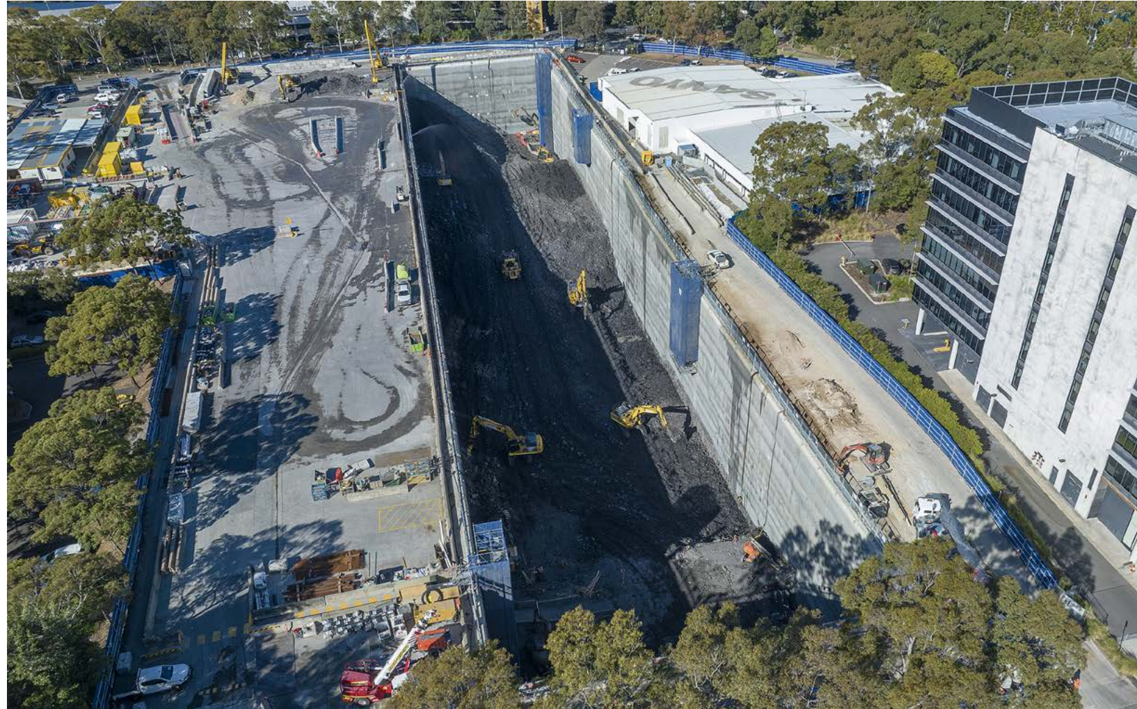
A bird's-eye view: Sydney Metro's new metro station at Sydney Olympic Park.
