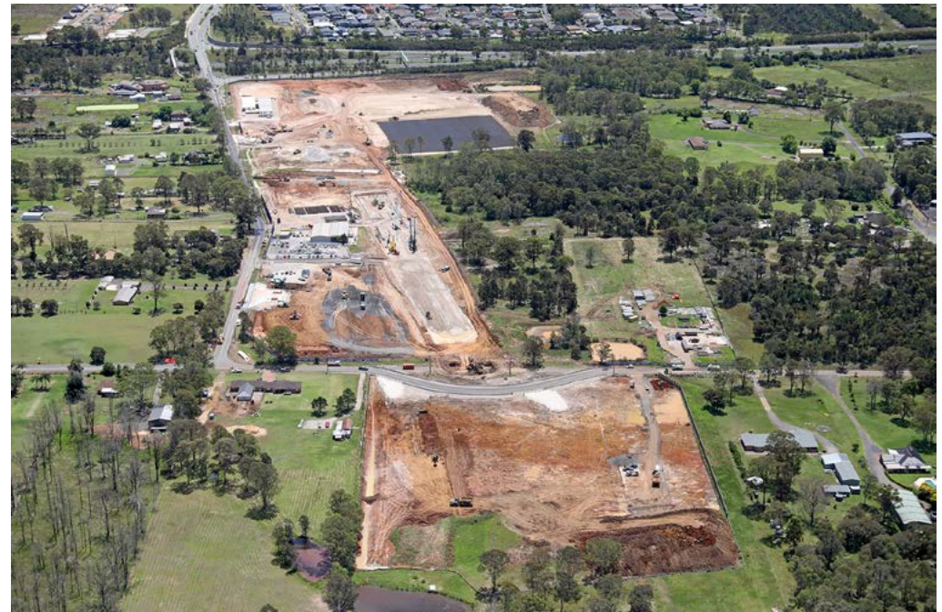
In progress: View of construction work at the new Orchard Hills Station, part of Sydney Metro – Western Sydney Airport.
