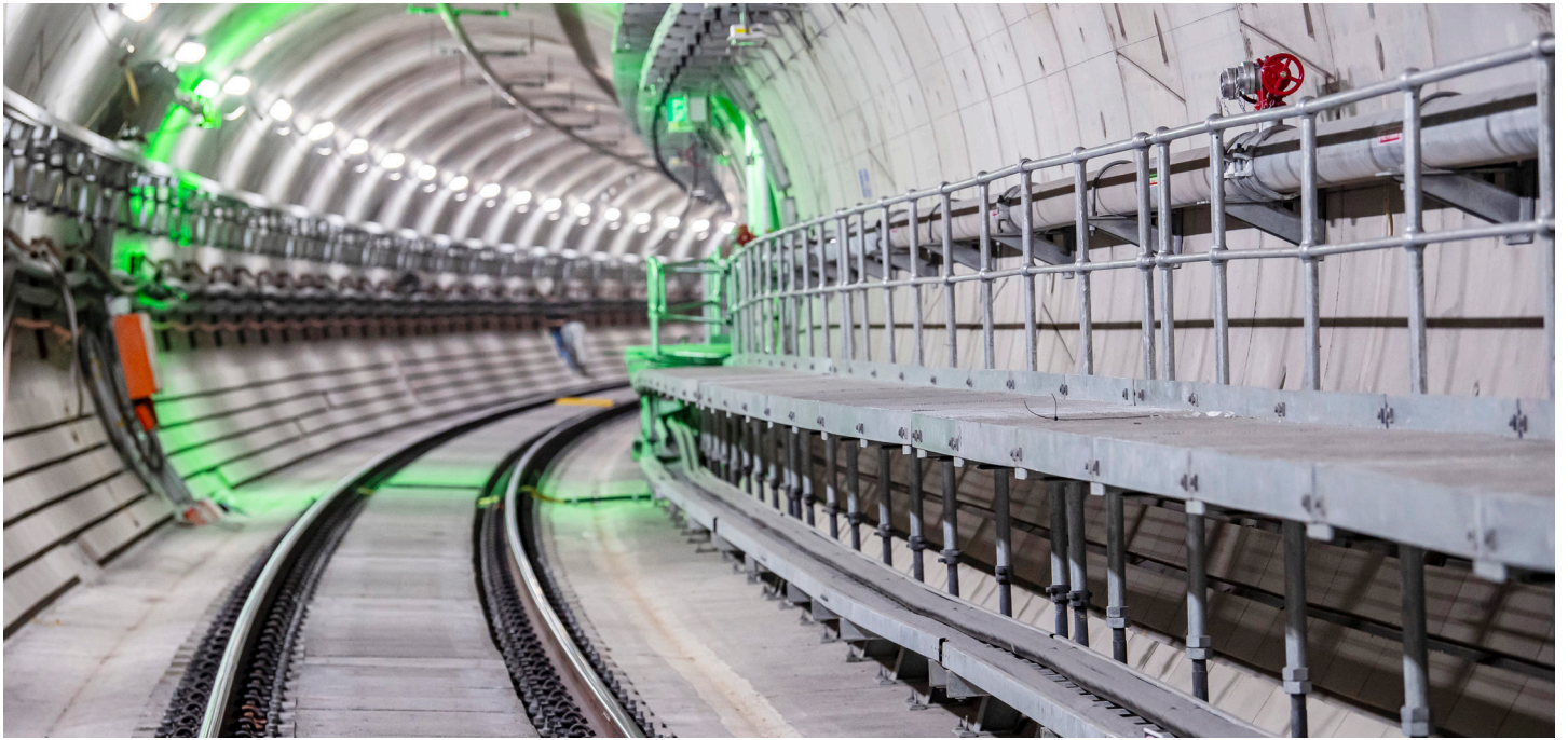
Below ground at Marrickville, the twin 15.5 kilometre tunnels to Chatswood are being prepared for energisation of the overhead wire.
