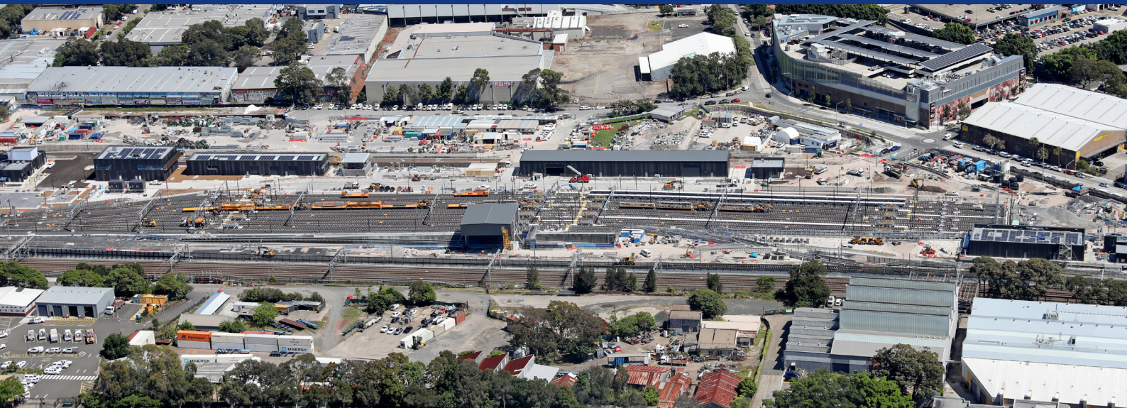
Construction of the stabling yard, services buildings and fit-out of the twin tunnels below ground, is nearing completion.
