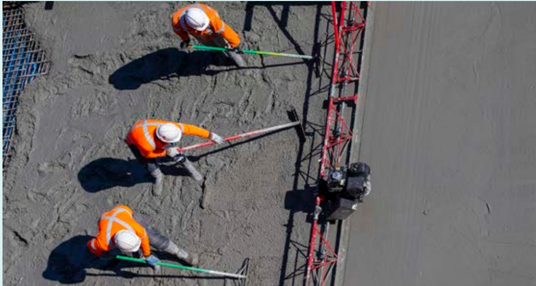
Concrete being poured at Barangaroo Station, part of Sydney Metro City & Southwest.
