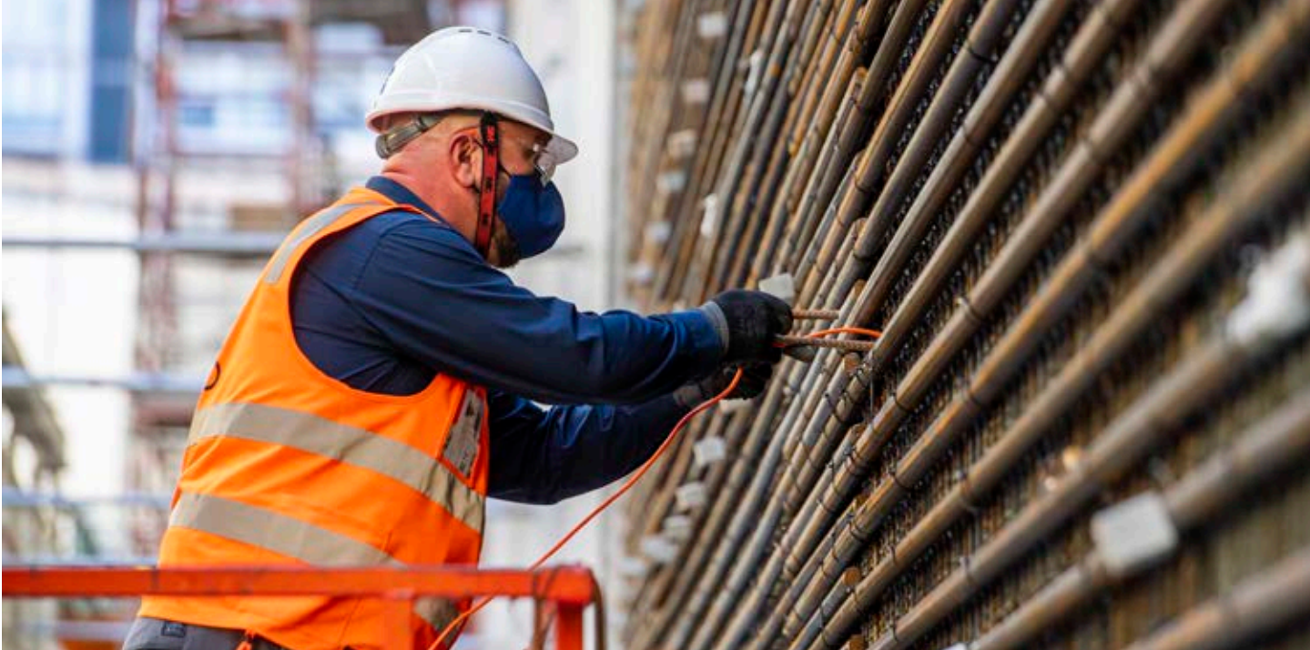
Construction work at Crows Nest Station, one of the new stations being built for Sydney Metro City & Southwest.
