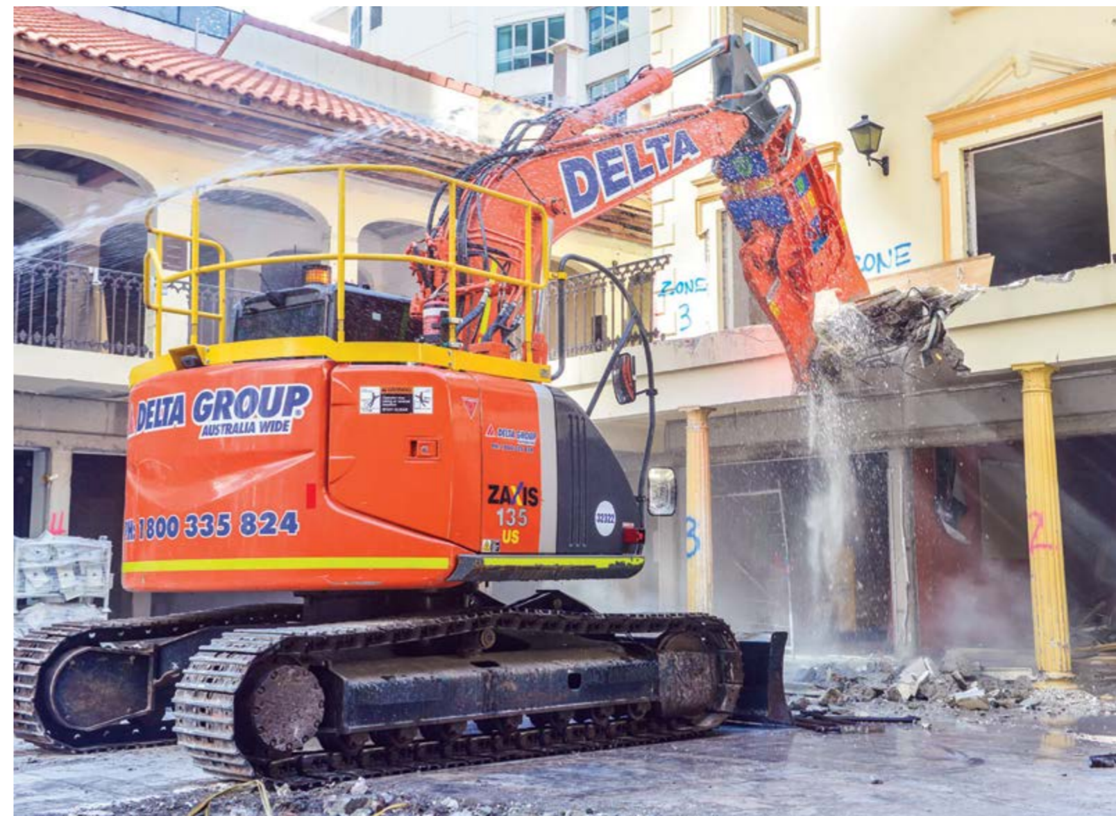
Pulveriser engaging in demolition works on the Sydney Metro City & Southwest project at Victoria Cross work site.
