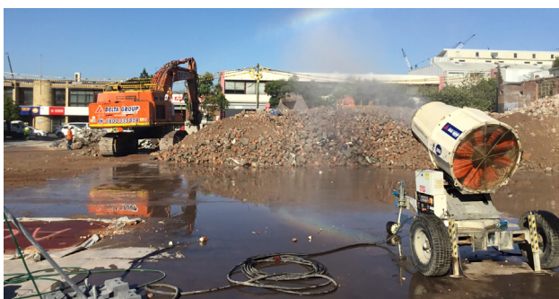
Misting cannon in use to control dust generation during load out of masonry waste.
